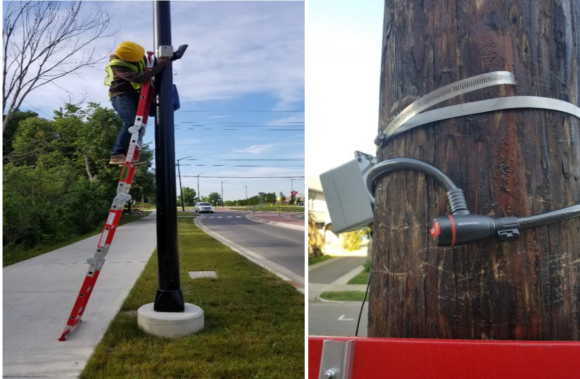
Figure 3.3: Installation of cameras on sites with bike lanes or shared lane markings
