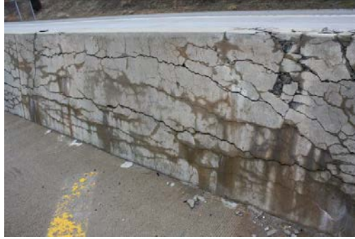
Figure 2.3-1. Example of ASR symptoms such as map cracking, cracks parallel to restraint, gel exudation, surface discoloration, etc. (Picture used with permission from Richard Deschenes).
