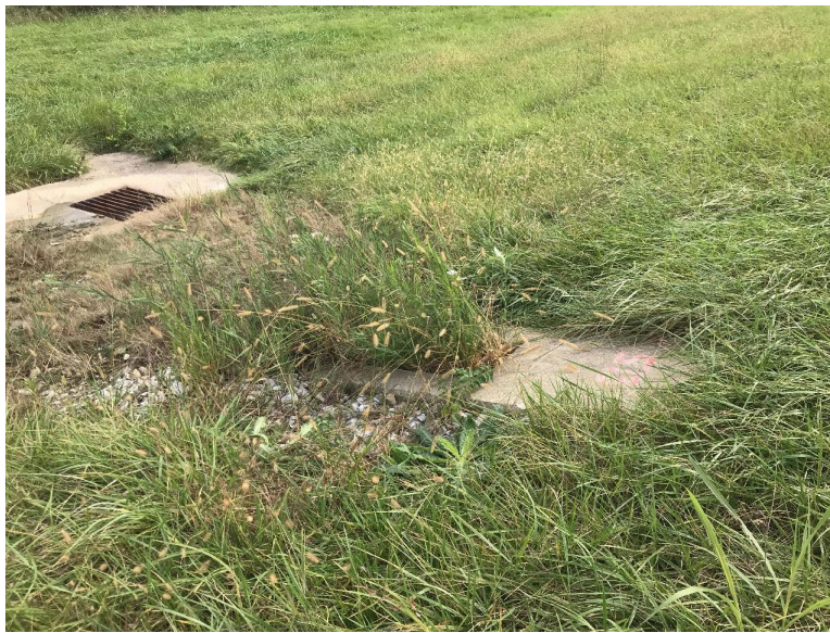
Figure 4 Outlet Waterway Blocked by Vegetative Growth
