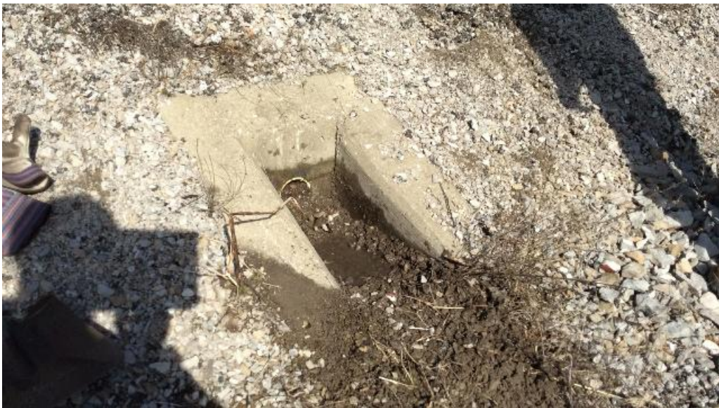
Figure 8 Blocked Outlet Pipe
