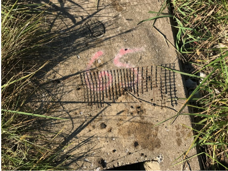
Figure 9 Rodent Screen Rusted Through
