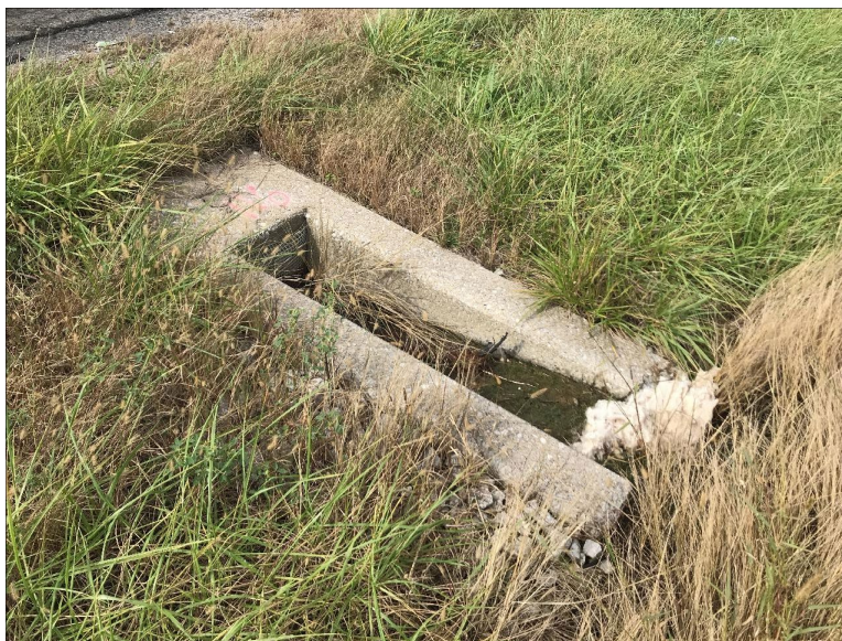
Figure 2 Outfall Waterway Obstructed by Debris
