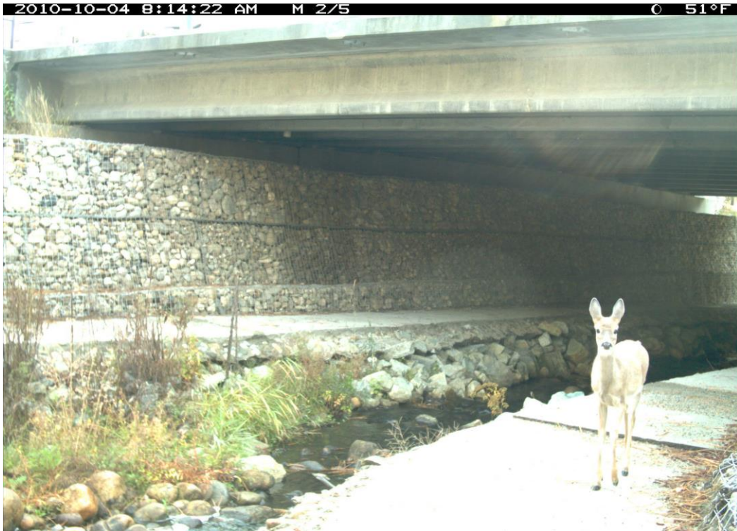
Figure 42. US 93 mp 70.5 Bass South Bridge, 4 (H) x 14 (W) x 27.4 (L) meters, 13 x 46 x 76 feet, Openness ratio (meters) 2.0.
