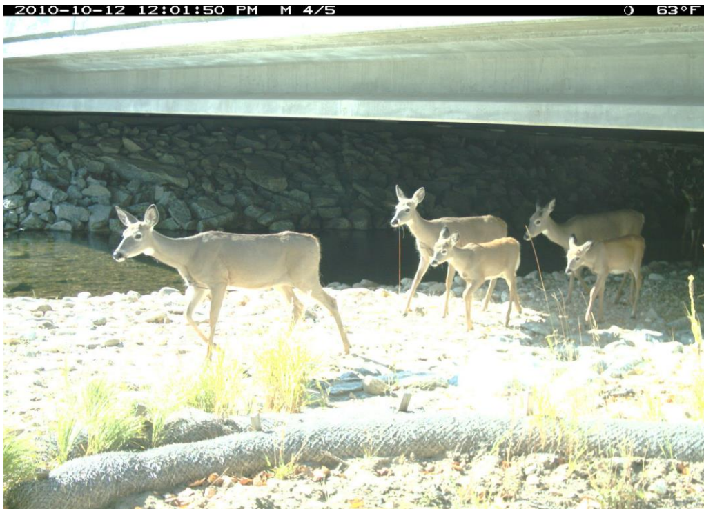
Figure 45. US 93 mp 66.2 Kootenai Creek Bridge, 1.8 (H) x 24 (W) x 27 (L) meters, 5.9 x 79 x 88.6 feet, Openness Ratio (meters) 1.6.
