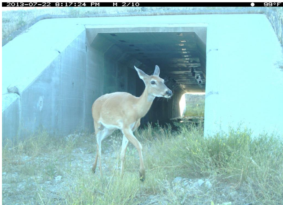
Figure 57. US 93 mp 56.2 Mountain Gallery Culvert, 2.7 (H) x 2.7 (W) x 54 (L) meters, 9 x 9 x 177 feet, Openness Ratio (meters) 0.14.
