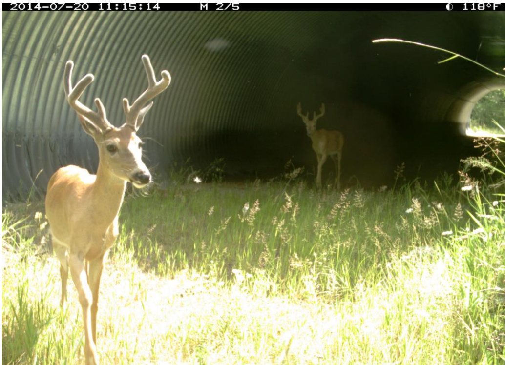
Figure 43. US 93 mp 70.1 Bass Fishing Access Culvert, 3.9 (H) x 6 (W) x 58 (L) meters, 12.7 x 20 x 190 feet, Openness Ratio (meters) 0.40.
