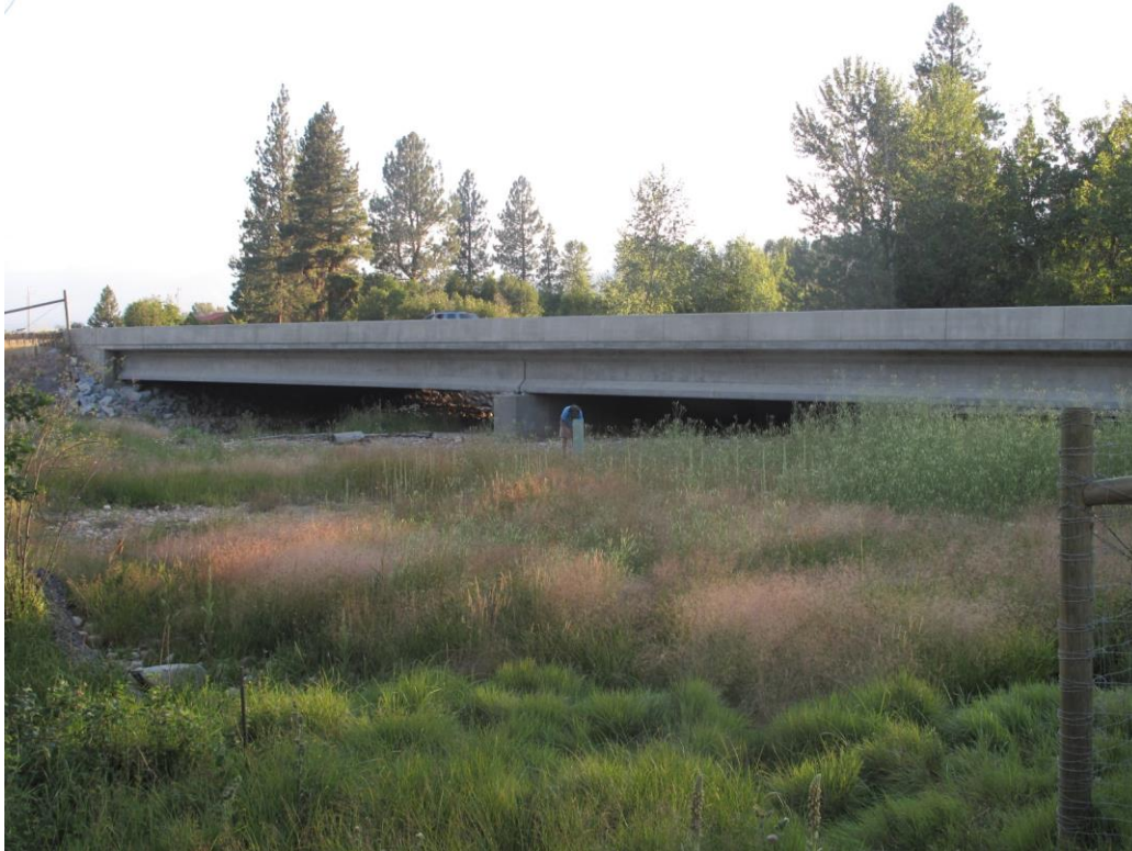
Figure 50. US mp 61.6 Big Creek Bridge, 1.4 (H) x 19 (W) x 26.5 (L) meters, 4.5 x 62 x 87 feet, Openness Ratio (meters) 4.3. View from Northeast Corner. Note Researcher Bent Over Camera Box in Foreground for Height Comparison.
