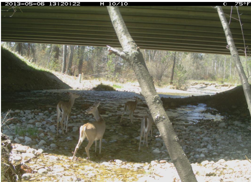
Figure 55. US 93 mp 57.1 Bear Creek South Bridge, 3.8 (H) x 36.3 (W) x 27.3 (L) meters, 12.5 x 119 x 89.5 feet, Openness Ratio (meters) 5.0.
