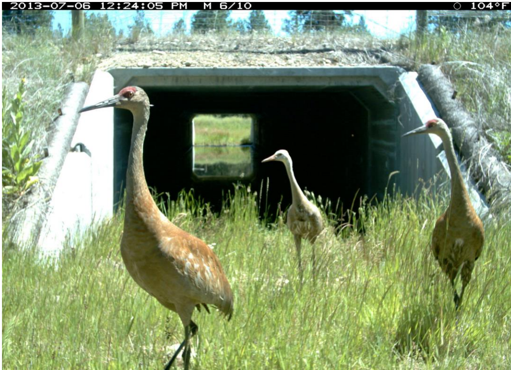
Figure 48. US 93 mp 64.6 Kootenai Springs Ranch Culvert, 2 (H) x 3.6 (W) x 44 (L) meters, 6.5 x 11.8 x 144 feet, Openness Ratio (meters) 0.16.
