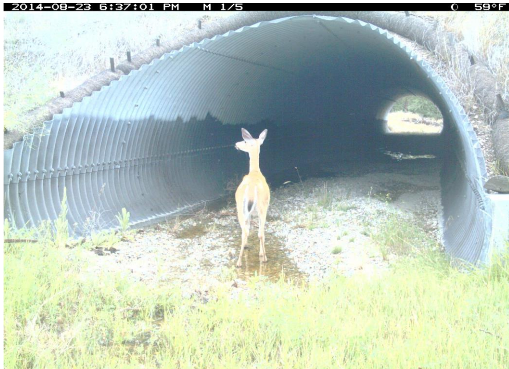
Figure 52. US 93 mp 60.7 Axmen Propane Culvert, 3 (H) x 4 (W) x 51 (L) meters, 9.8 x 13 x 161 feet, Openness Ratio (meters) 0.24.
