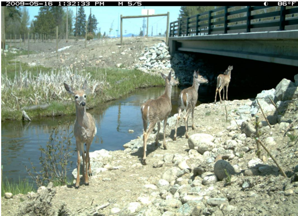
Figure 46. US 93 mp 66.1 McCalla North Bridge, 1.9 (H) x 24 (W) x 26.4 (L) meters, 6 x 79 x 86 feet, Openness Ratio (meters) 1.7.
