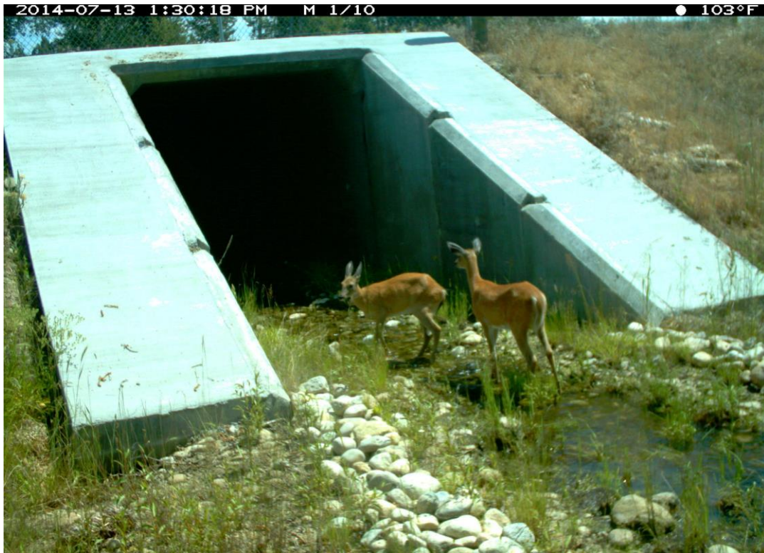
Figure 56. US 93 mp 56.7 Lupine Culvert, 2.7 (H) x 2.7 (W) x 52 (L) meters, 9 x 9 x 170 feet, Openness Ratio (meters) 0.14.
