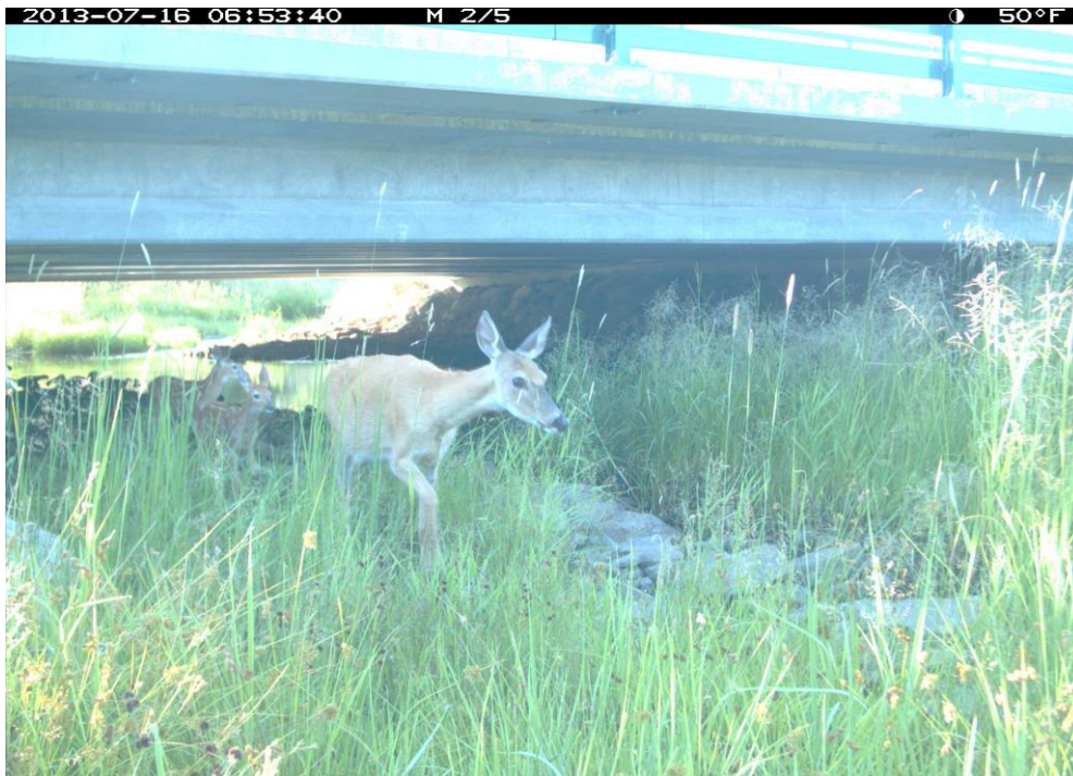
Figure 47. US 93 mp 65.1 McCalla South Bridge, 1.4 (H) x 19 (W) x 26.5 (L) meters, 4.5 x 62 x 87 feet, Openness Ratio (meters) 1.0.
