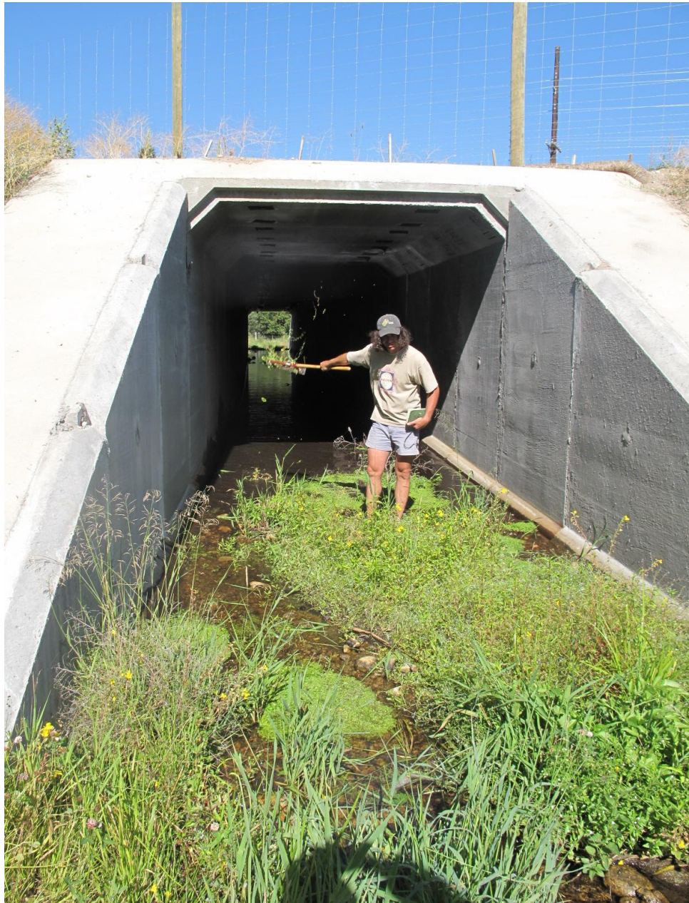
Figure 58. US 93 mp 55.5 Fun Park Culvert, 2.7 (H) x 2.7 (W) x 58 (L) meters, 9 x 9 x 190 feet, Openness Ratio (meters) 0.13.
