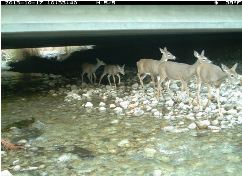
Figure 54. US 93 mp 58.3 Bear Creek North Bridge, 1.3 (H) x 21 (W) x 27.4 (L) meters, 4.3 x 69 x 90 feet, Openness Ratio (meters) 1.0.
