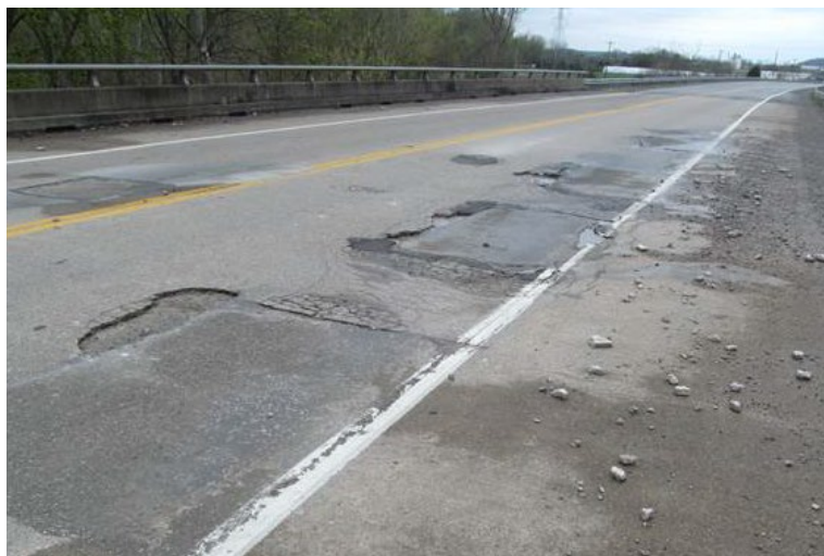
Figure 1 Damage Observed on Bridge Decks
