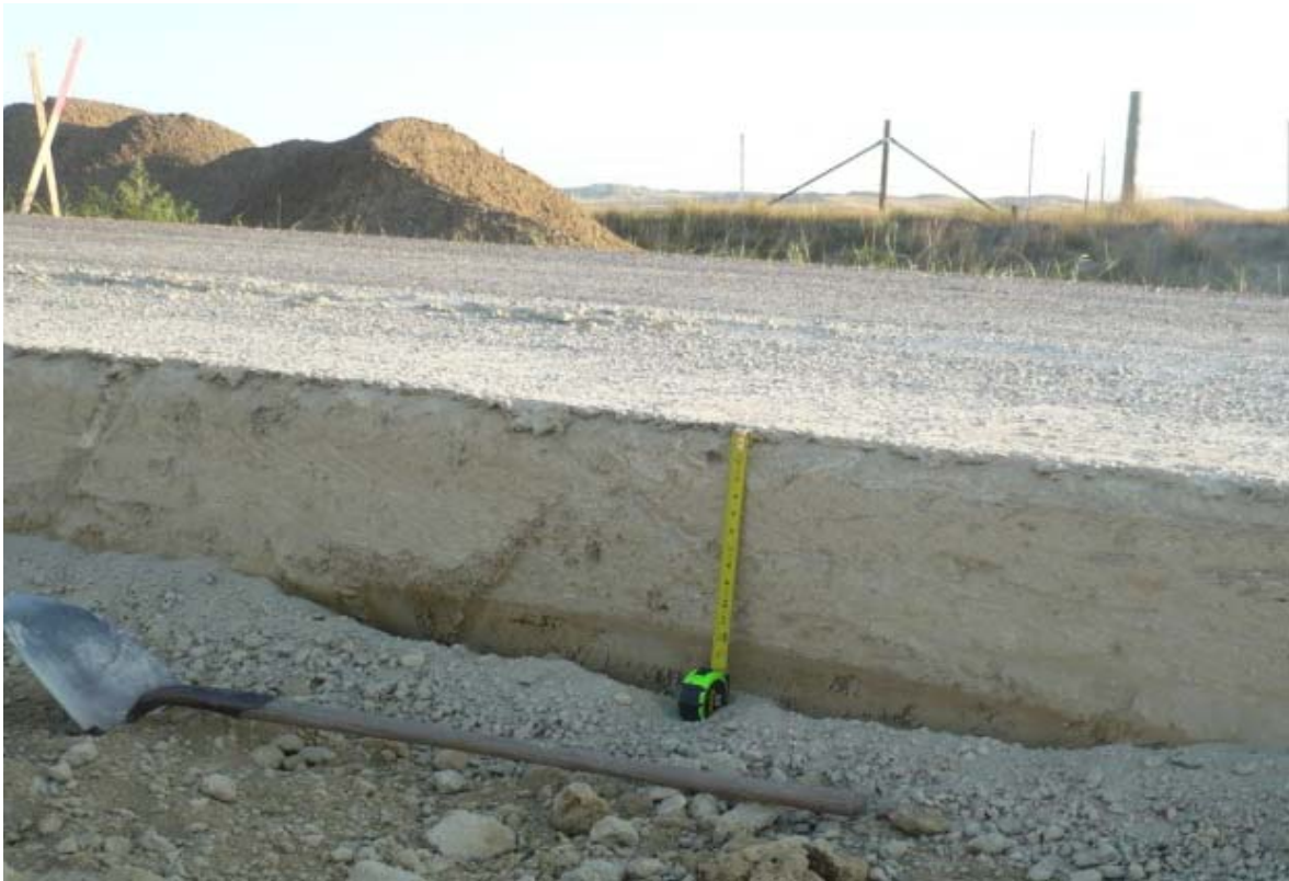
FIG. 3. Twelve inch thick soil cement layer with Double BST on surface and moist underlying clay subgrade (2012 repair of 2011 soil cement on CR 146E).
