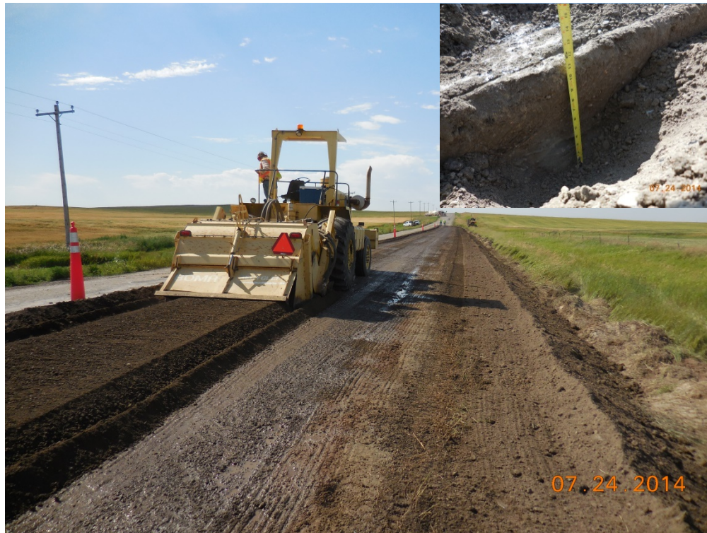
FIG. 20. Full Depth Reclamation (FDR) of Soil Cement to 12 inch depths with the addition of 3% more Portland cement.
