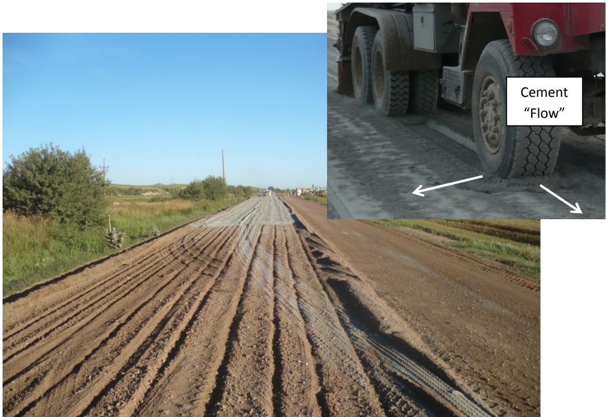
FIG. 23. Cement spread placement and alignment controlled by berms along road shoulder and centerline. Road surface ripping prior to cement spreading reduces cement “flow” caused by water truck and pulverizer/mixer tires.
