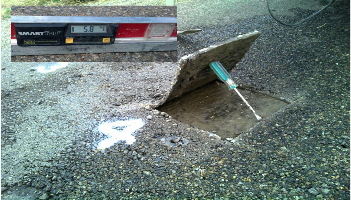
FIG. 13. Clean chip BST on paving fabric, CR 321N. Note lack of adhesion and significant lateral movement on soil cement surface. Photo insert shows road crown measurement of 5.8 percent, almost two percent over the specification limit.
