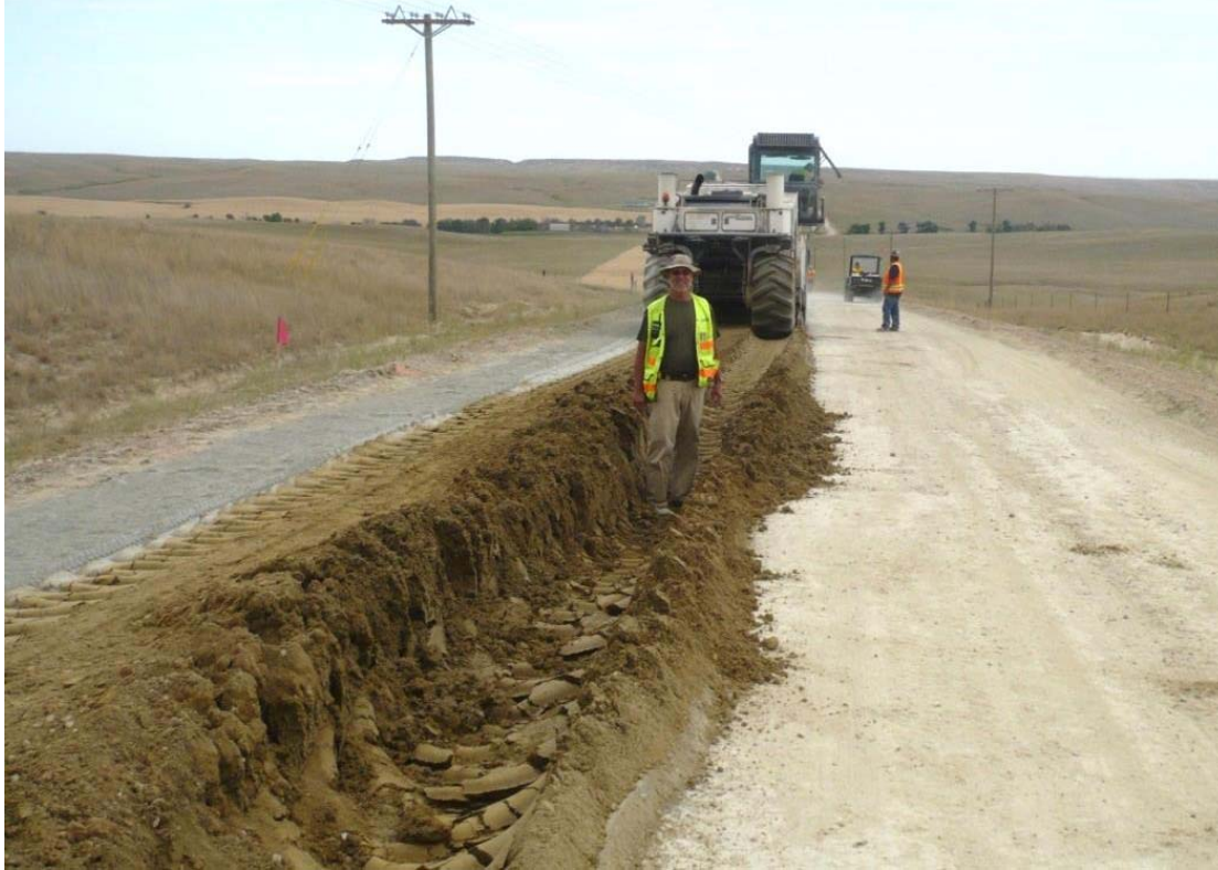
FIG. 28. Sandy silt wet area from perched water table close to road centerline.
