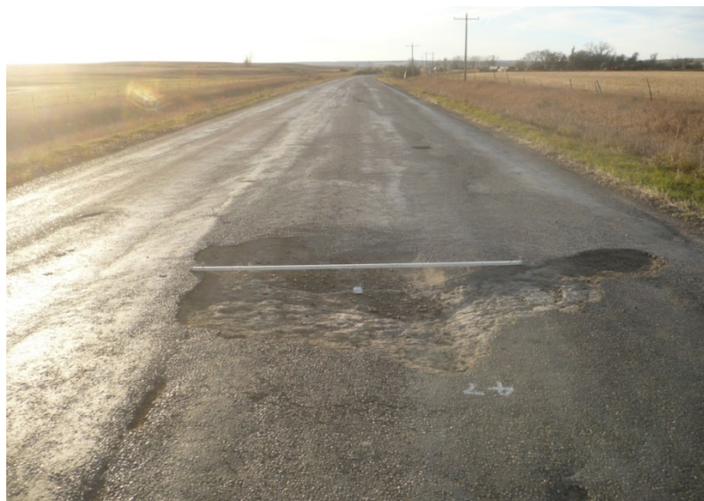
FIG. 18. Pothole location coincides with transverse joint location. Pothole caused by either low cement content, pulverization, moisture content or compaction. White straight edge is 2.4 m (eight feet) long and 25 mm (one inch) square.
