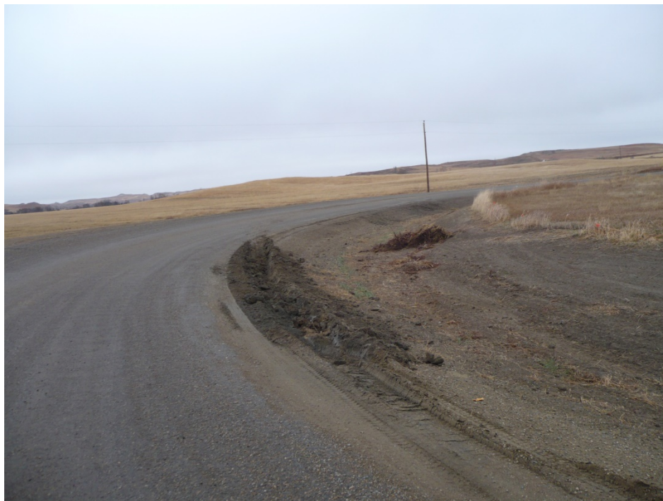
FIG. 22. Weak shoulders outside the 28 foot wide subgrade soil stabilization.
