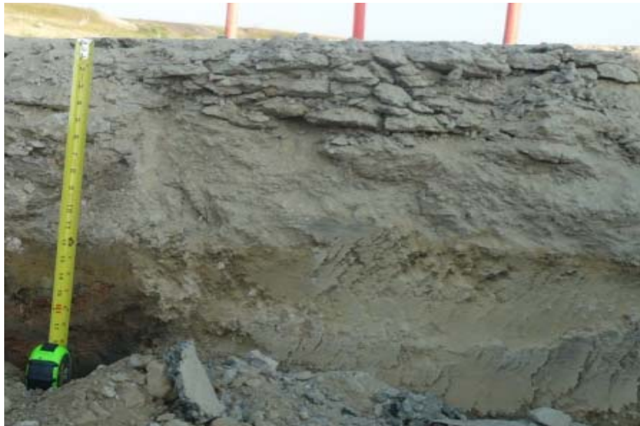
FIG. 16. Wheel track cracking (rubbleization) of 300 mm (12 inch) thick soil cement layer.
