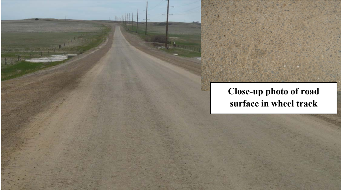
FIG. 4. Treated gravel surface containing 3.5% Bentonite clay and 1.5% dry calcium chloride. Percentages are based on dry weight of aggregate.
