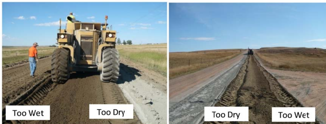
FIG. 26. Unacceptable moisture uniformity primarily due to internal spray bar plugging caused by inadequate mixing chamber cleaning.
