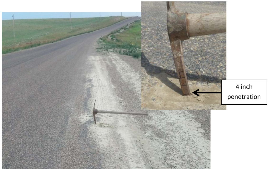
FIG. 24. Pick axe probe to determine if sufficient cement was used in rutted areas. Photo was taken six months after stabilization. Pick penetrated 50 mm (2 inches) into dense clay – no strength from cement was evident in soil chunks.
