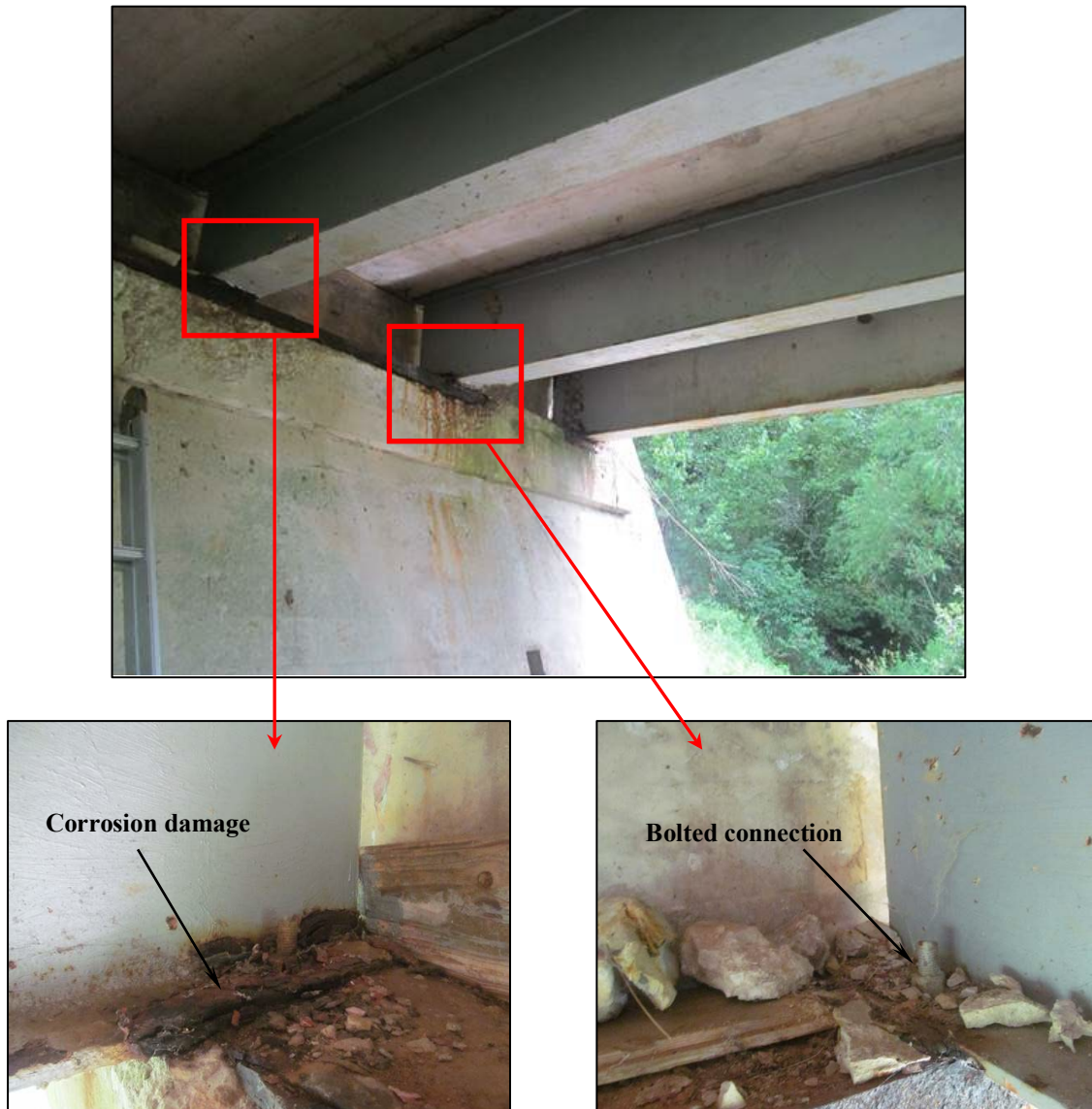
Fig. 18 Bottom flange connection and typical corrosion at beam ends
