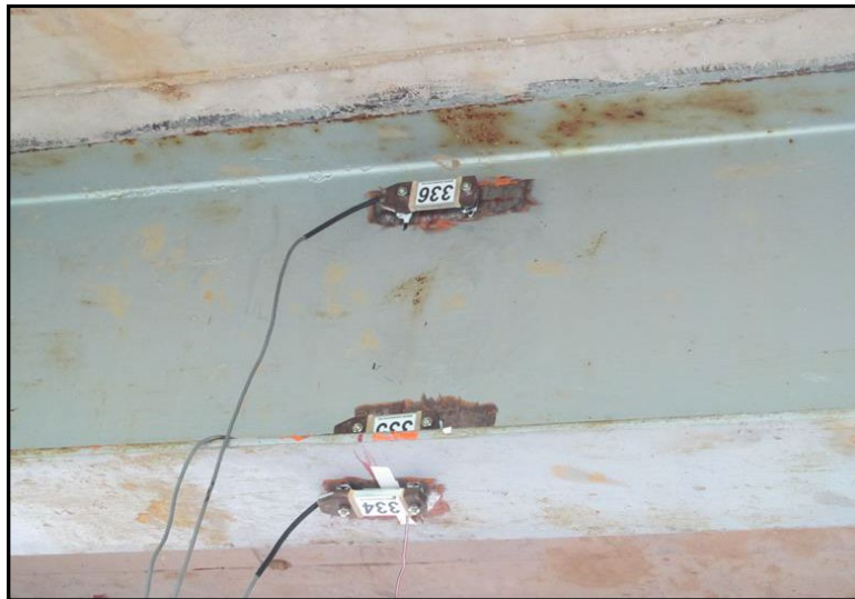
Fig. 19 Strain gauges on interior beam
