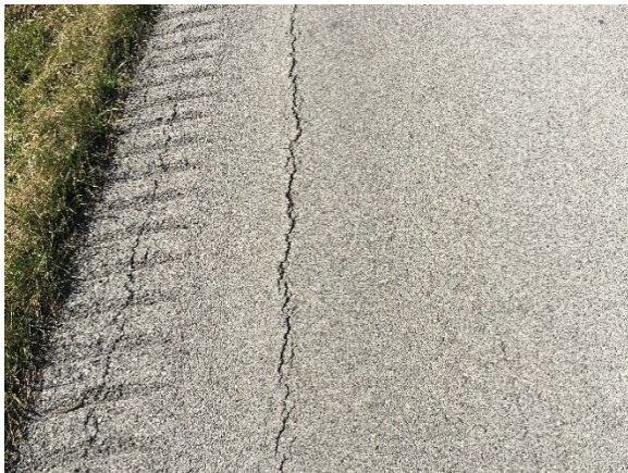
Figure 35. Moderate Longitudinal Crack
