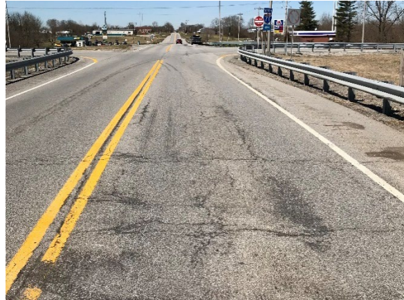
Figure 42. Heavy Cracking and Raveling
