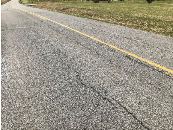
Figure 25. Heavy Longitudinal Cracking
