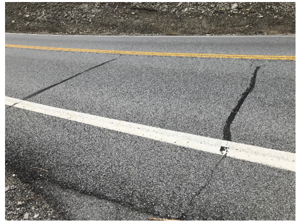
Figure 22. Sealed Transverse Cracks
