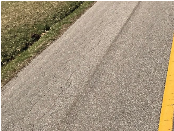
Figure 31. Base Failure Outside Edge
