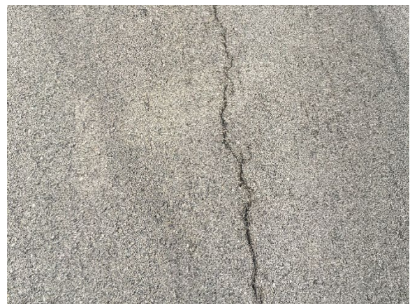
Figure 40. Moderate Longitudinal Cracking
