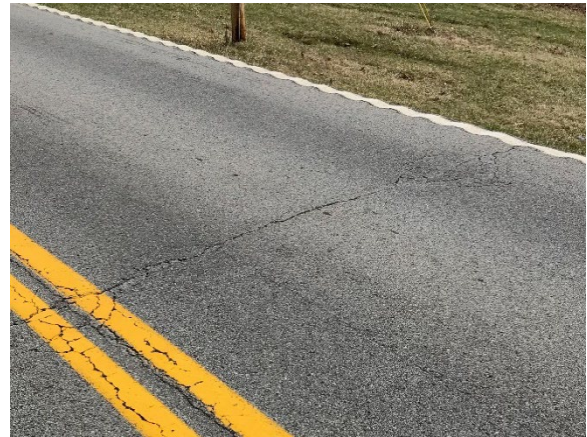
Figure 48. More Transverse Cracking
