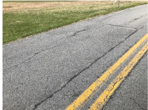
Figure 26. Patched (Cracking Again)
