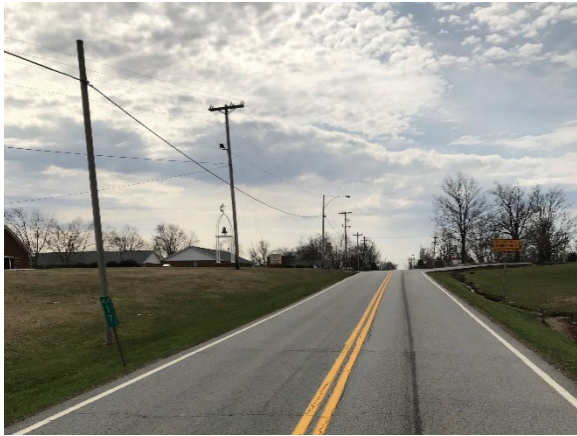
Figure 19. More Transverse Cracking
