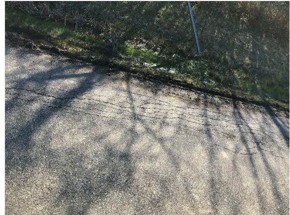
Figure 2. Base Failure Outside Edge
