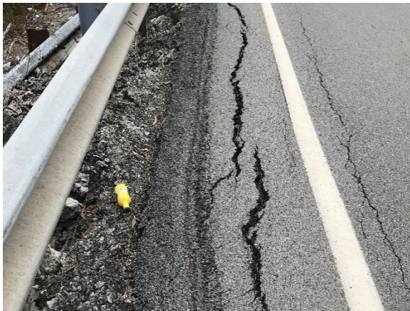
Figure 23. Moderate Base Failure
