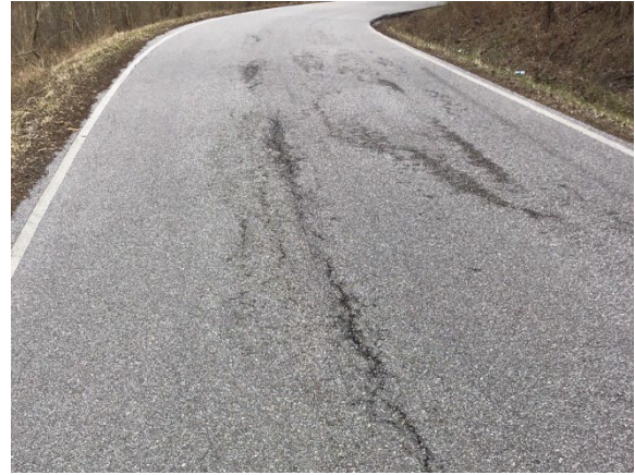
Figure 6. Moderate Cracking Across Lane
