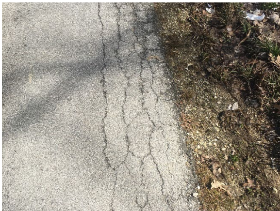
Figure 39. Bases Failure Outside Edge
