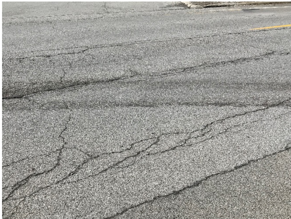
Figure 41. Heavy Longitudinal Cracking
