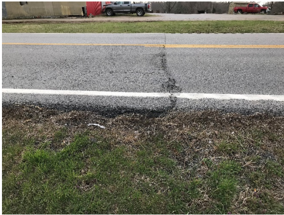
Figure 47. Moderate Transverse Cracking
