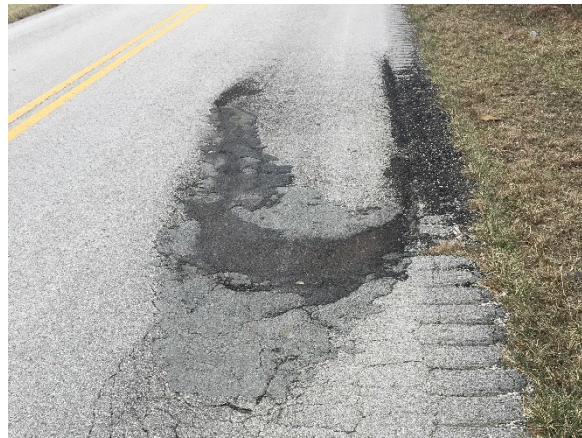
Figure 11. Severe Base Failure with Patching
