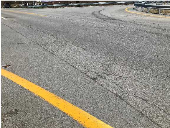
Figure 43. More Heavy Cracking
