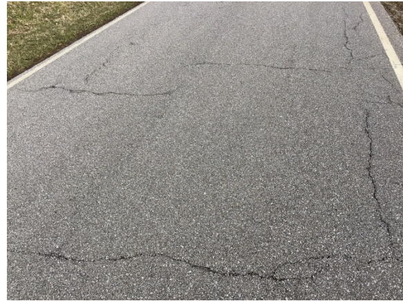
Figure 8. Transverse & Longitudinal Cracks
