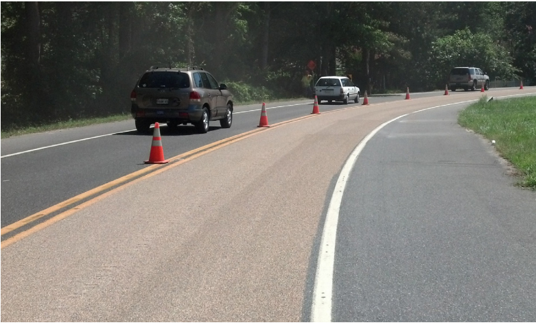
A section of high-friction surface treatment applied in Delaware cures before the road is opened to traffic.
