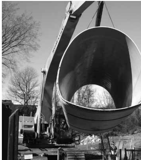
Innovative technologies used for a sewer rehabilitation project in Clifton, New Jersey, resulted in a $1.4-million savings.
