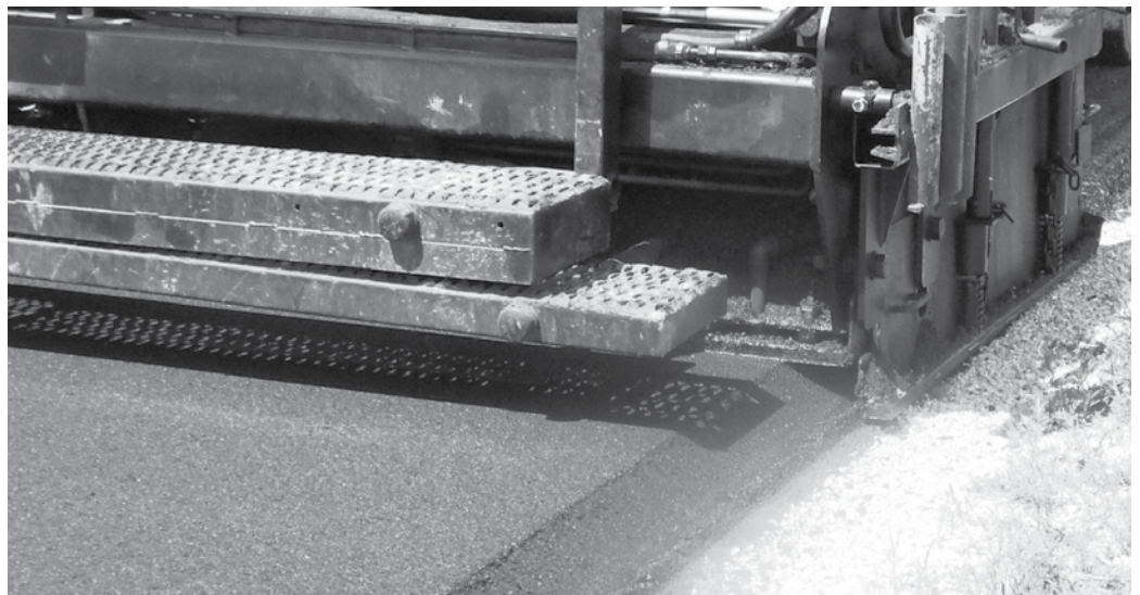
The Safety Edge is a paving technique where the edge of the pavement is shaped to approximately 30 degrees.
