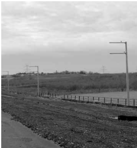
The Texas Department of Transportation used developer-managed and owner-managed utility relocation agreements for the construction of State Highway 130.
