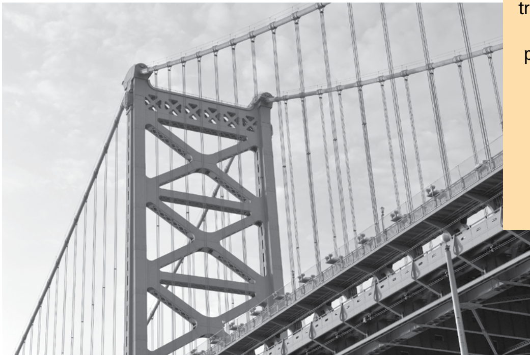
FHWA's new Bridge Construction Inspection course discusses an inspector's safety responsibilities and potential hazards that an inspector may encounter.
