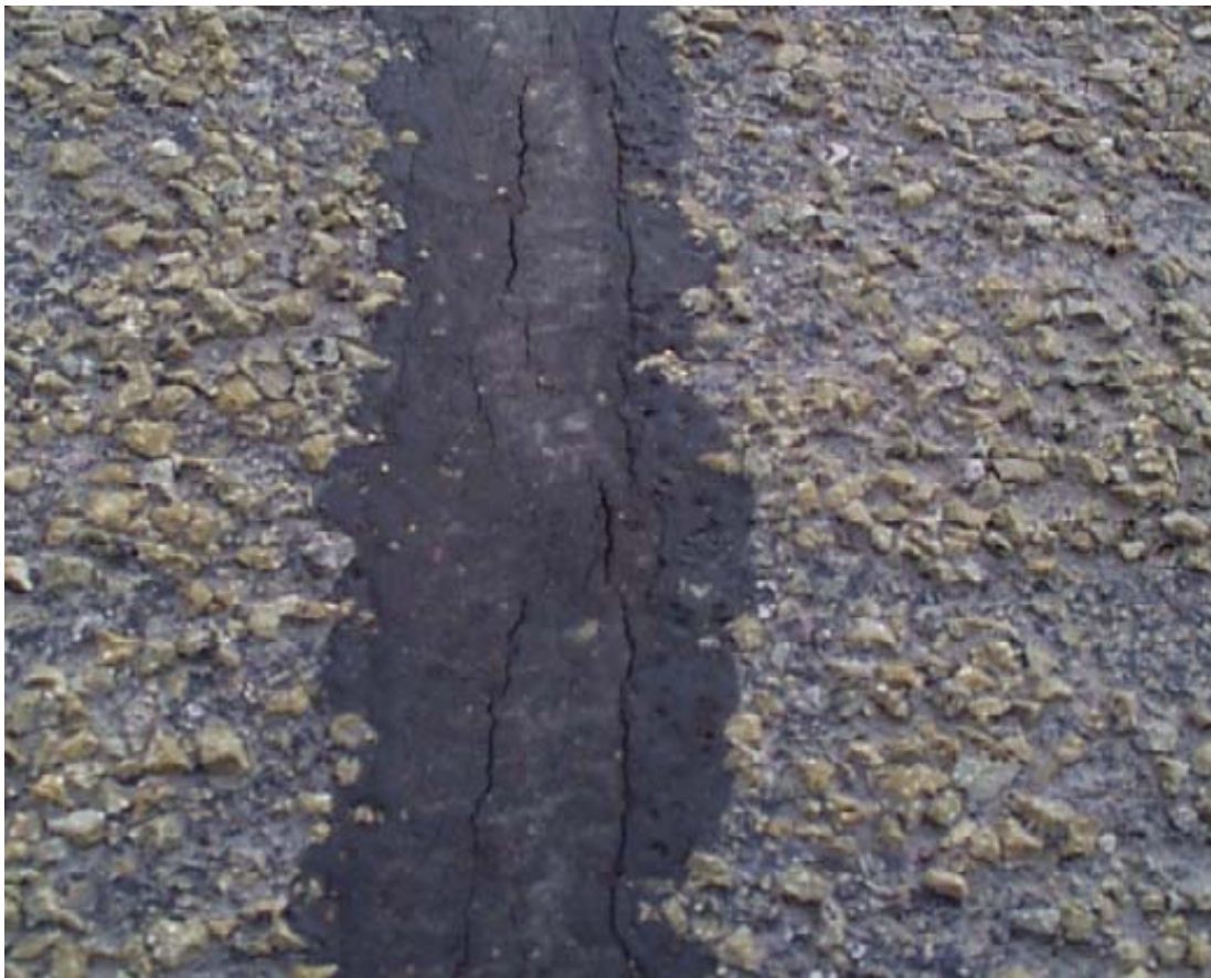
Figure 5: Example of Double Adhesion Failure Associated with the Shallow and Flush Technique
