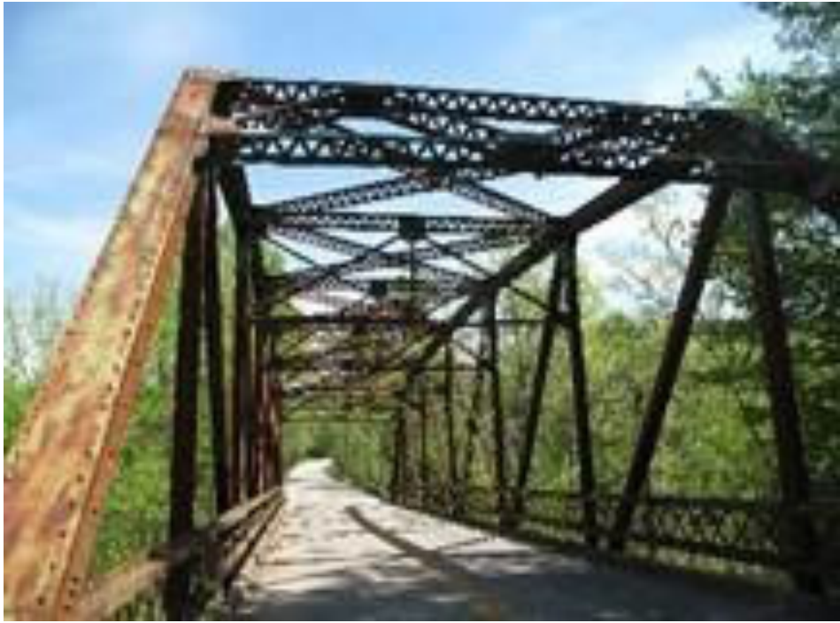
Figure A77: Jellico Creek Bridge Summary Sheet
