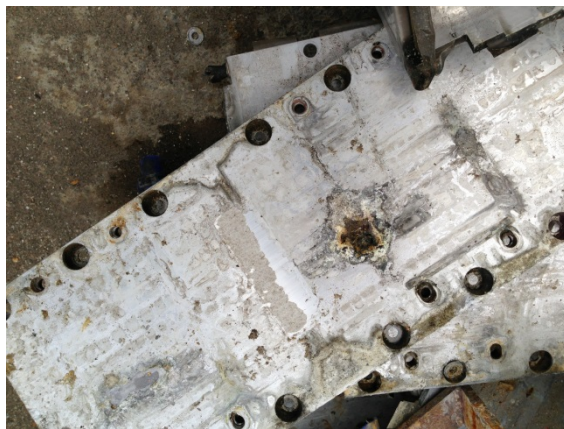
Figure 24: Evidence of arcing/aggressive discharge
