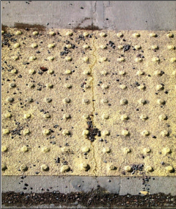
Installation 5B: Close-up of mortar crack through mat.
