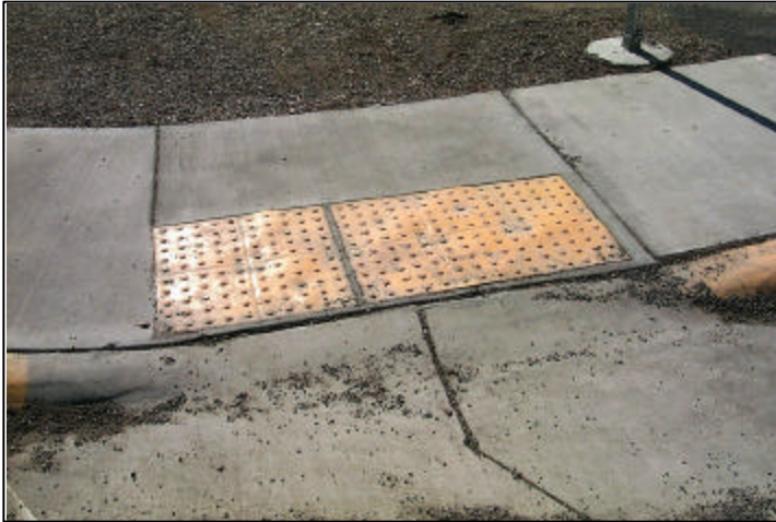
Installation 2: Located on the southwest corner at the intersection of 6 th Ave. N. W. and 6 th St. N. W.
