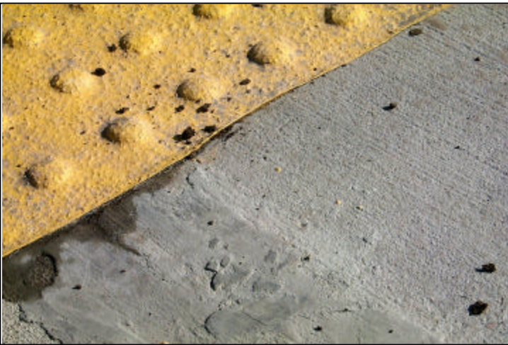
Installation 6A: Example close-up of edge losing adhesion from PCCP.
