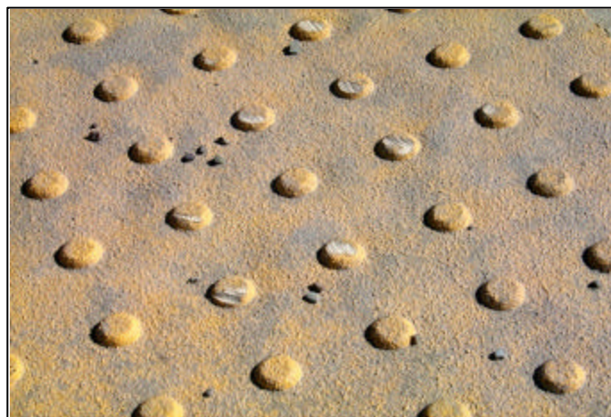
Installation 7: Additional close-up of damaged mat. Sheared domes from blade damage.
