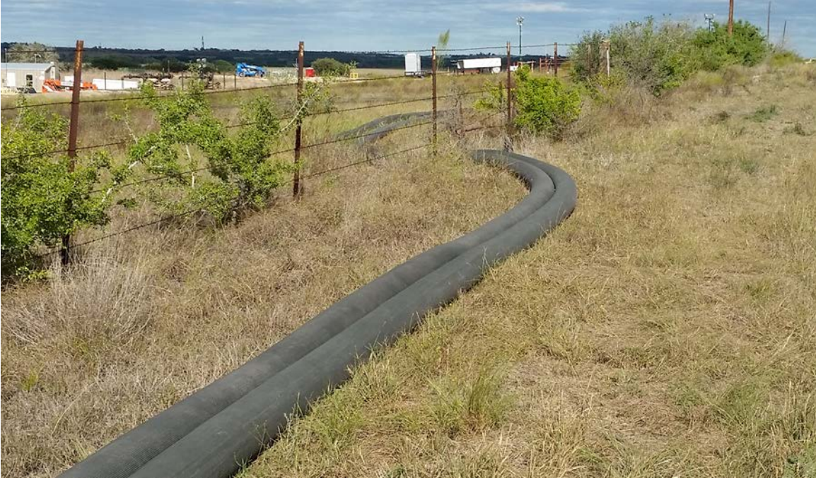
Figure 24. Temporary Pipelines Crossing Right-of-Way Line without Signage.
