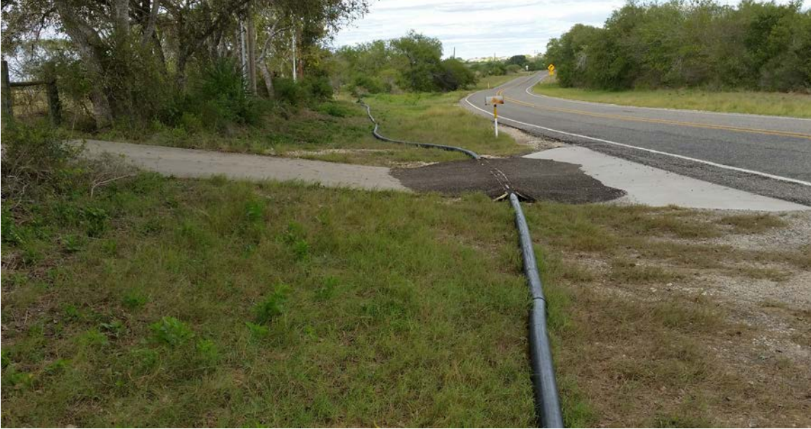
Figure 18. Temporary Pipeline Ramp Installed at Low Point of Right of Way with Asphalt Transition.
