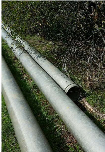
Figure 8. Aluminum Temporary Pipelines.
