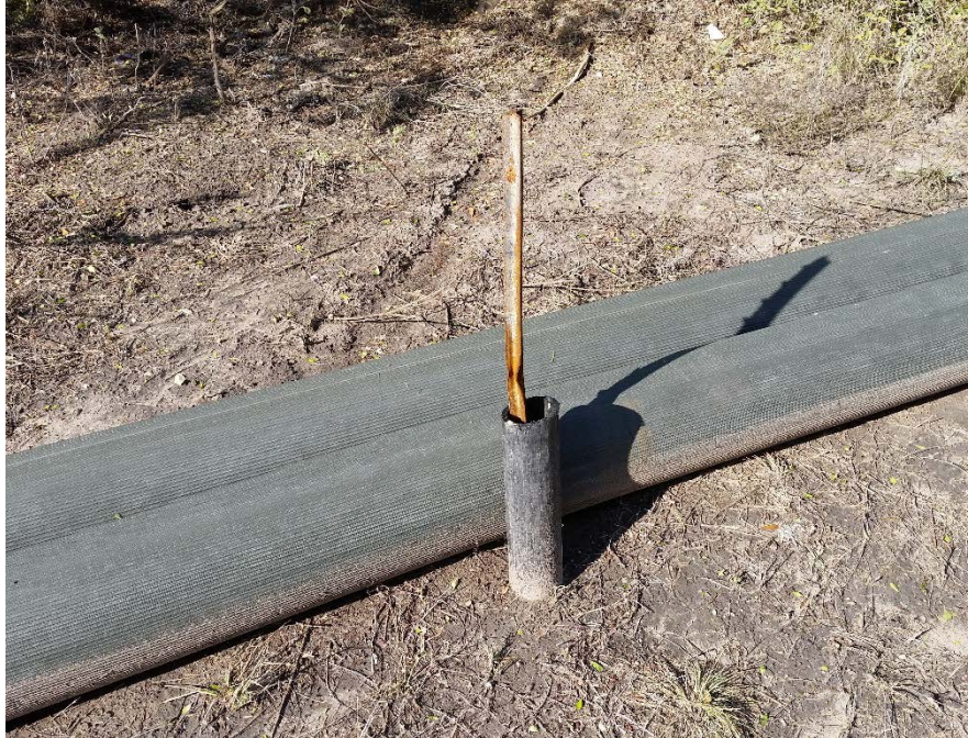
Figure 10. Protective Sleeve between Stake and Temporary Pipeline.
