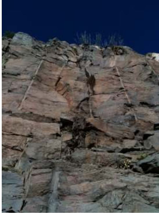
Figure 10. Rock slope in Scan 2 showing pre-split half-casts, blasting fractures, and natural fractures.
