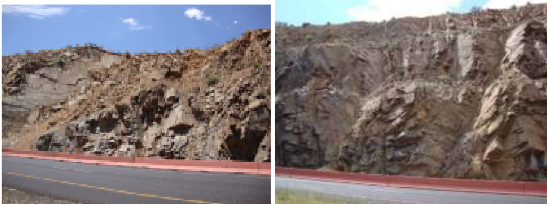
Figure 68. Wedge failures at the Texas site formed by discontinuity Sets 1 and 4 (see Figure 66b and Table 34).
