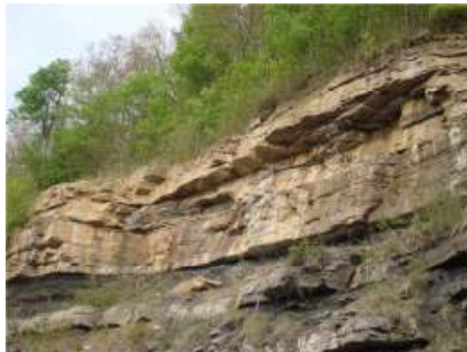
Figure 59. Photo of overhangs present on I-24 slope.
