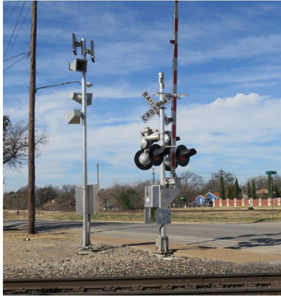
Figure 26. Automated Wayside Horn
