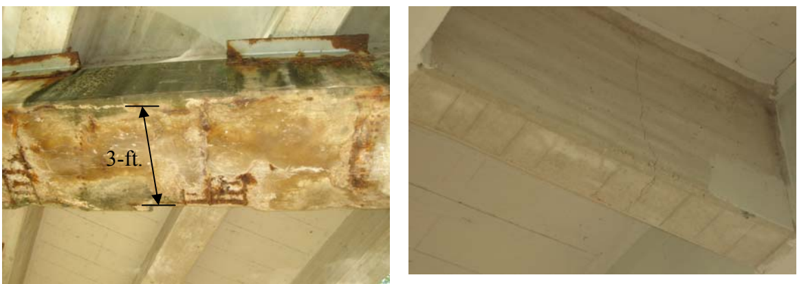
Figure 7.12. Bridge T-530 Corrosion of Bents and Cracked Transverse Beam
