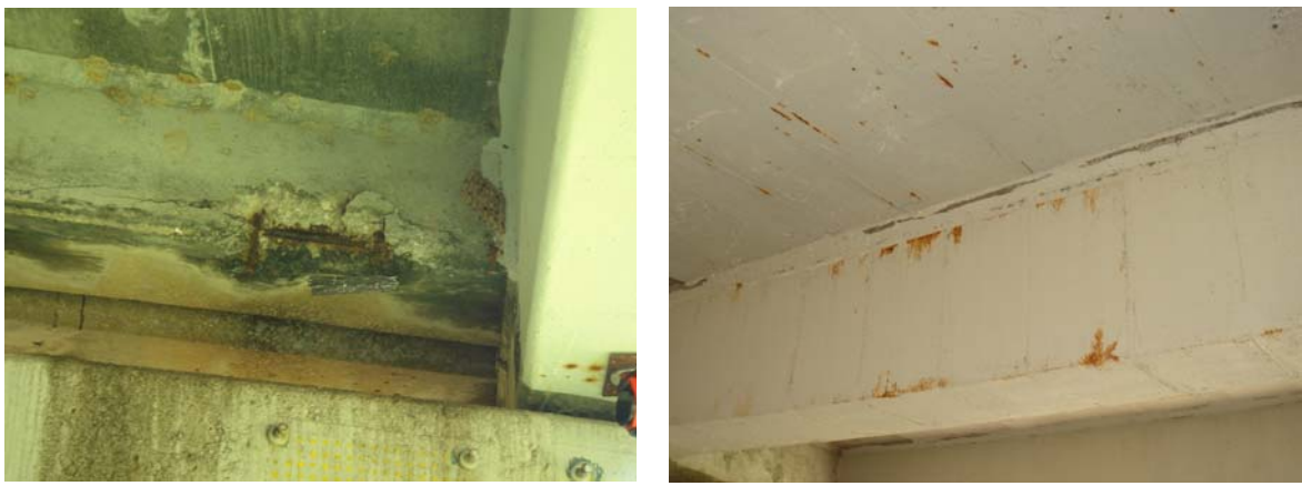
Figure 7.15. Bridge P-962 Corrosion of Transverse Girder and SRP Reinforcement
