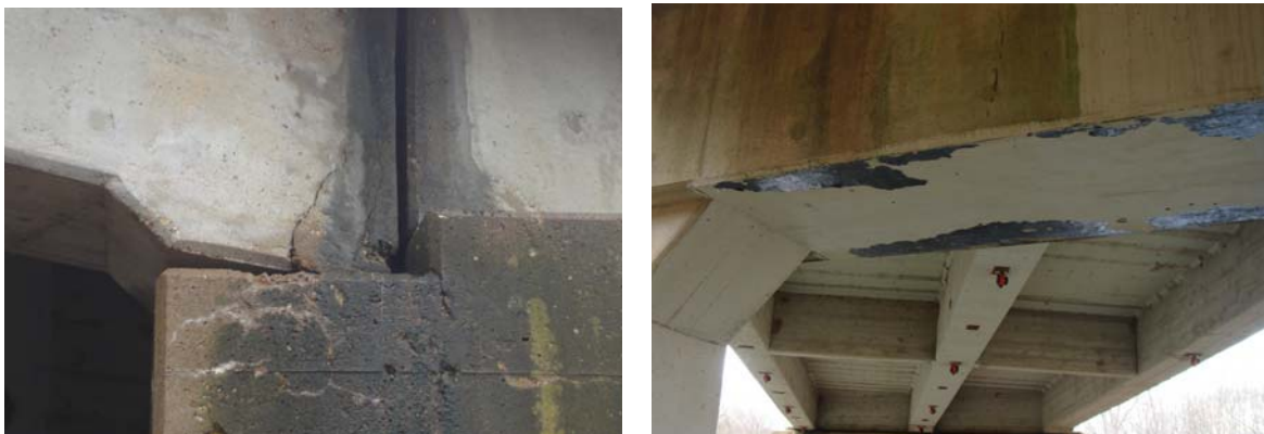
Figure 7.14. Bridge X-495 Disturbed Region Crack and Peeling of Protective Coating
