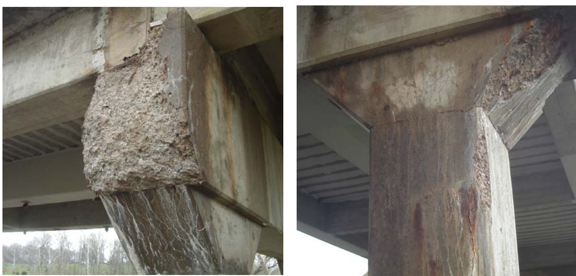
Figure 7.13. Bridge X-596 Corrosion of Bents
