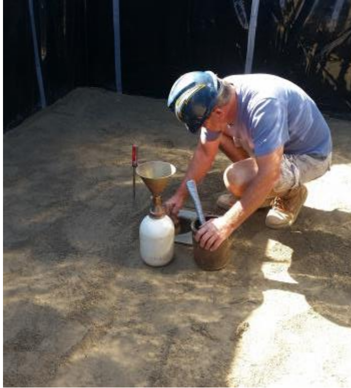
Figure A-9: Verification of the achieved soil density during backfilling from sand cone test
