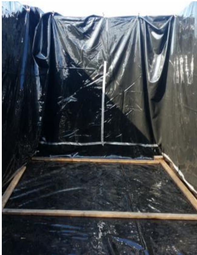
Figure A-4: Plastic lining inside the laminar soil container (the wood was removed during backfill)
