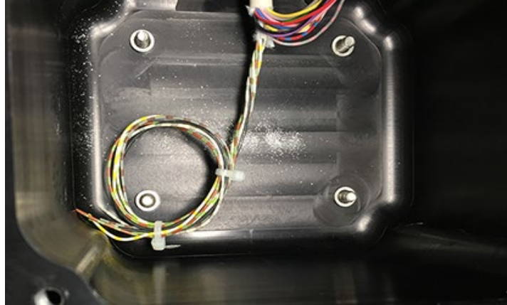
Figure 17. The silver powder-like crystals shown inside of the throttle control box are aluminum shavings from the detent housing caused by wear from the control lever's steel ball bearing
