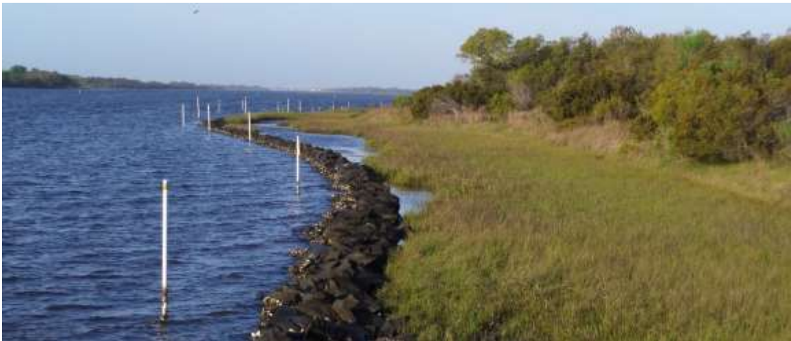
Figure 5-2. Stone sill and constructed marsh at Morris Landing, NC (photo courtesy of Bret Webb).
