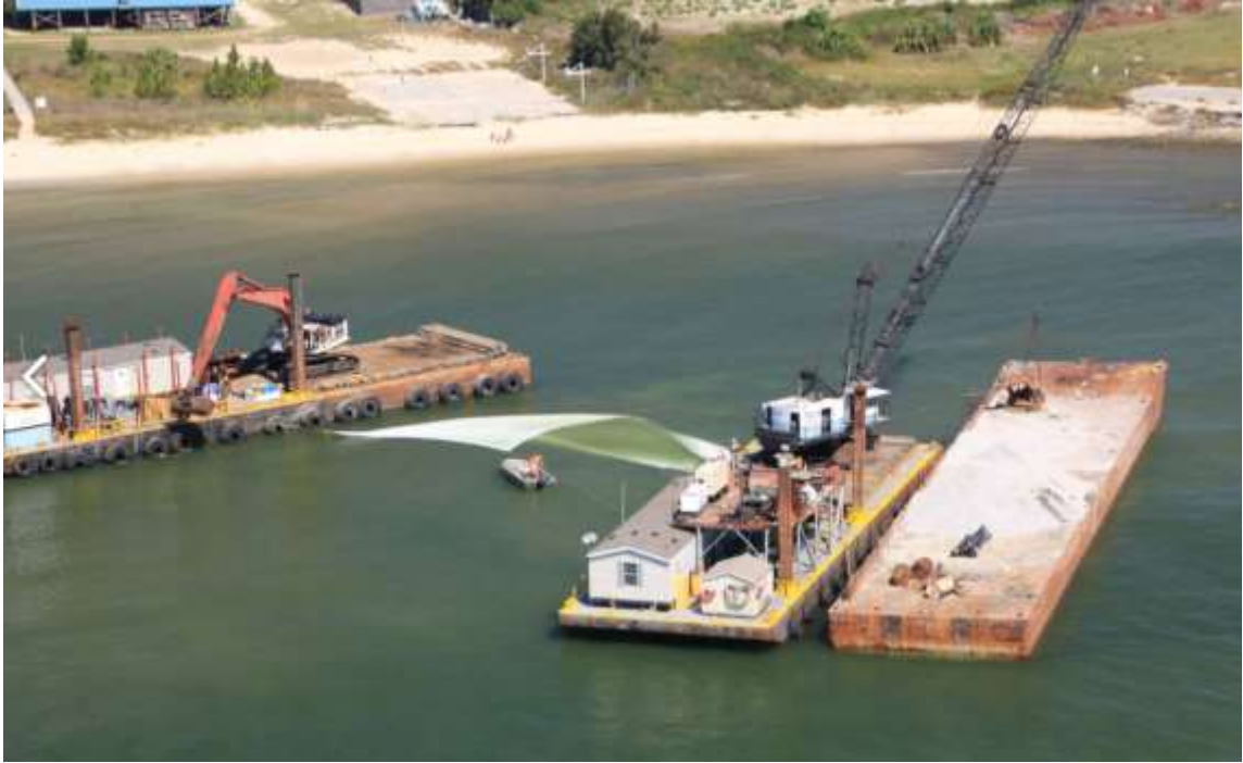
Figure 5-10. Contractors placing geotextile fabric for the foundation of an offshore rock breakwater (photo courtesy of Sam St. John).
