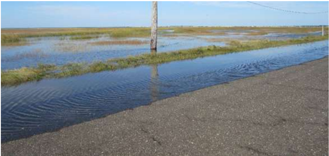
Figure 2-3. Flooding of Great Bay Boulevard during high tide (FHWA 2018c).
