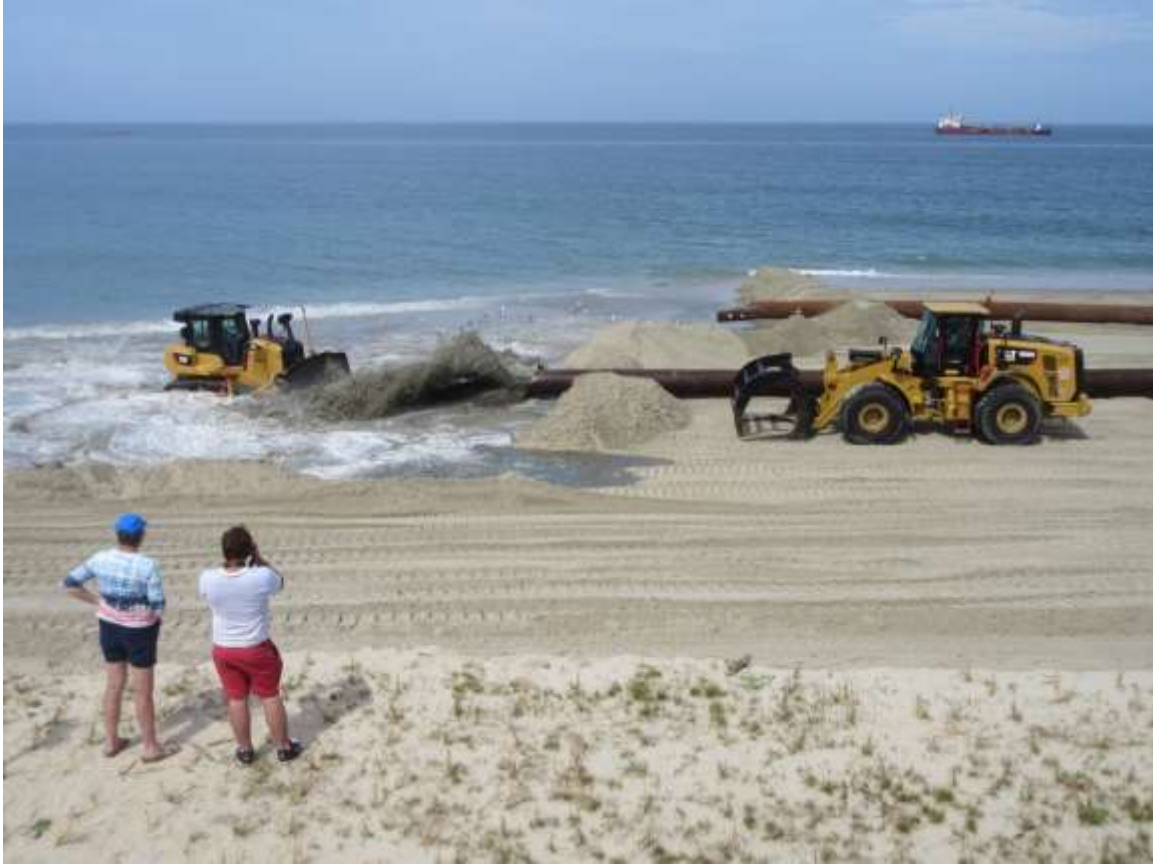
Figure 5-12. Active beach nourishment in North Carolina showing the dredge pipeline discharging sand and water directly onto the shore. The dredge ship is visible in the background (photo courtesy of Tina Hodges).
