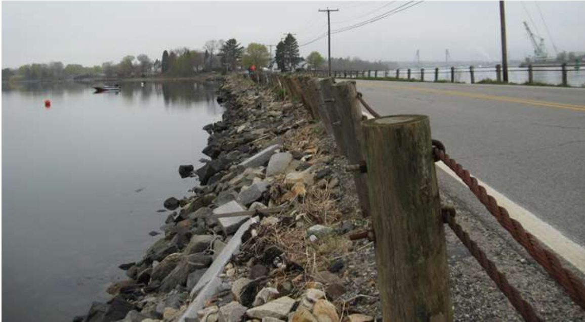
Figure 4-6. U.S. Route 1B causeway in New Castle, NH (photo courtesy of New Hampshire DOT).
