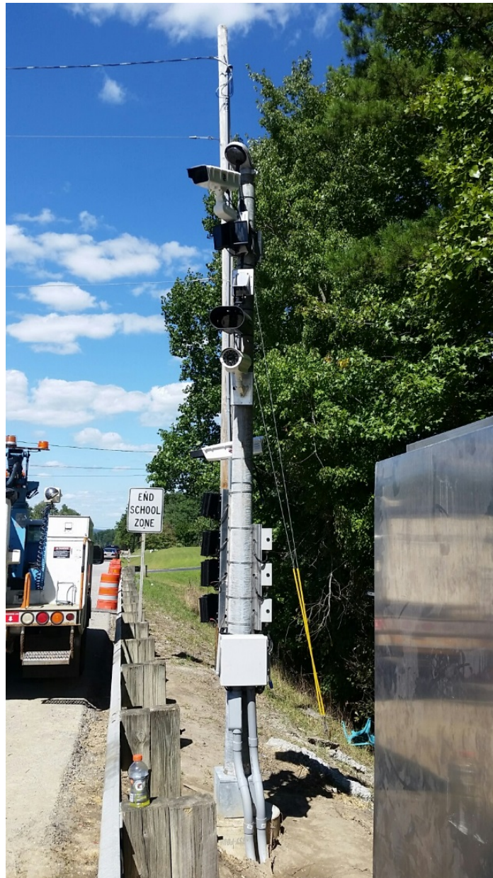
Figure 7. Photo. Laurel County, Tennessee virtual weigh station installation. (Source: FHWA)
