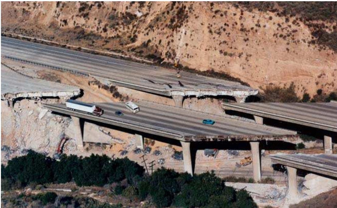
Figure 14. I-5 damage at Gavin Canyon (Source: Caltrans)
