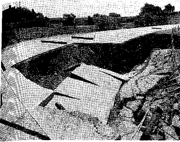
Fig. L - Pavement collapse before use
