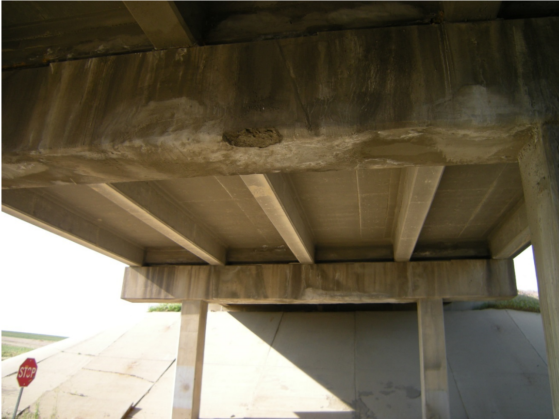
Figure 3.7 Discoloration under expansion joint on C-17-AT (photo courtesy CDOT)
