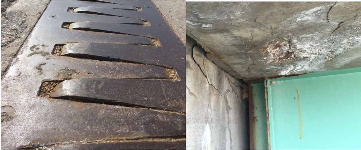
Figure 5.8 Deterioration of B-16-FM abutments and joints
