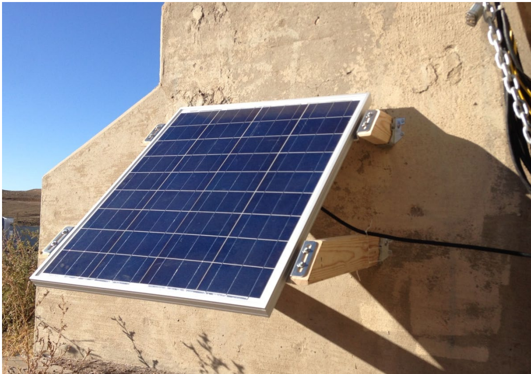
Figure 3.32 Solar panel attached to abutment
