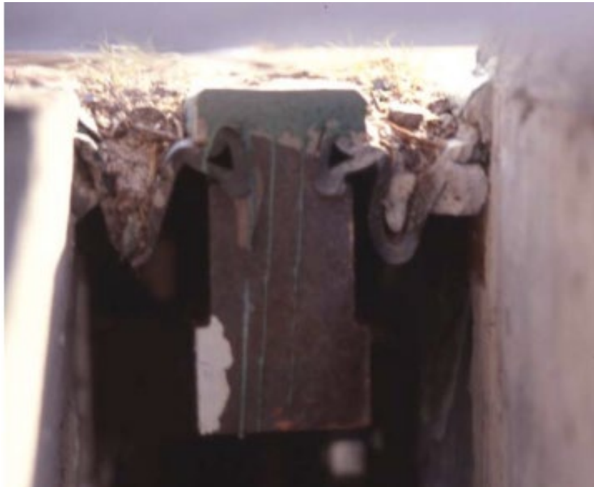
Figure 2.2 Debris in expansion joint in service for less than six months (Chen, 2008)
