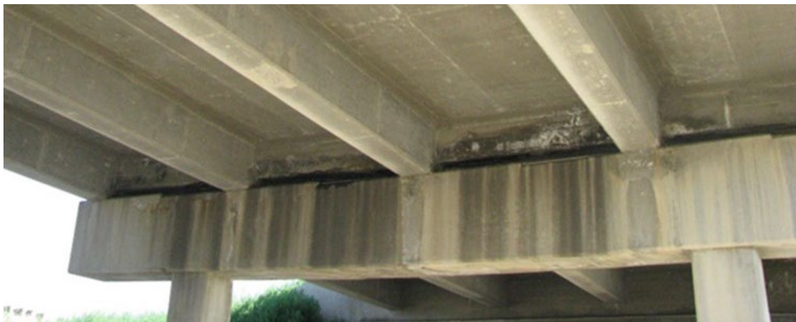
Figure 3.10 C-17-AT underside – corrosion and leakage
