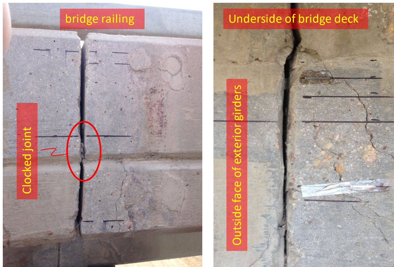
Figure 3.11 C-17-AT expansion joint clogging
