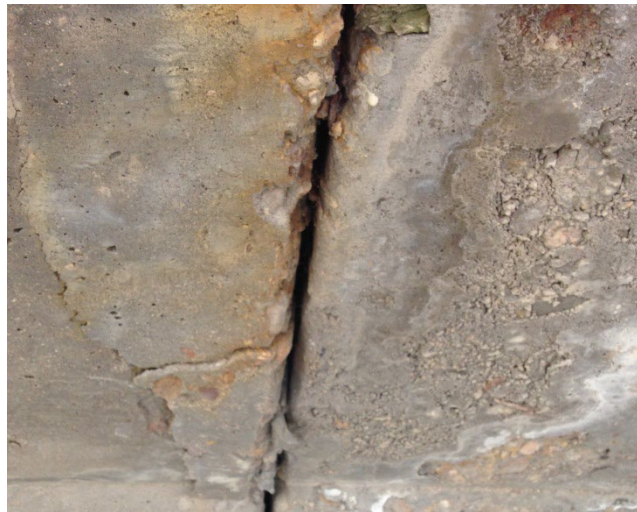
Figure 5.7 Deterioration of C-17-AT abutments and joints
