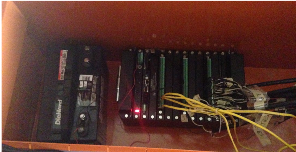
Figure 3.26 DAQ in job box
