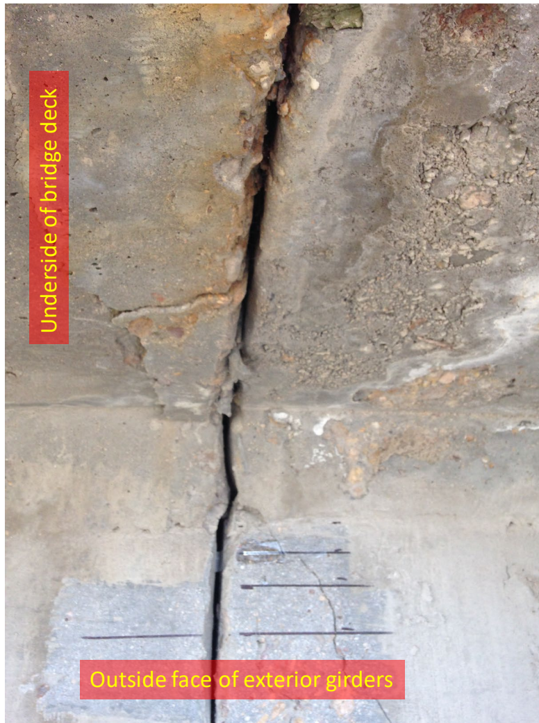
Figure 3.12 C-17-AT expansion joint deterioration
