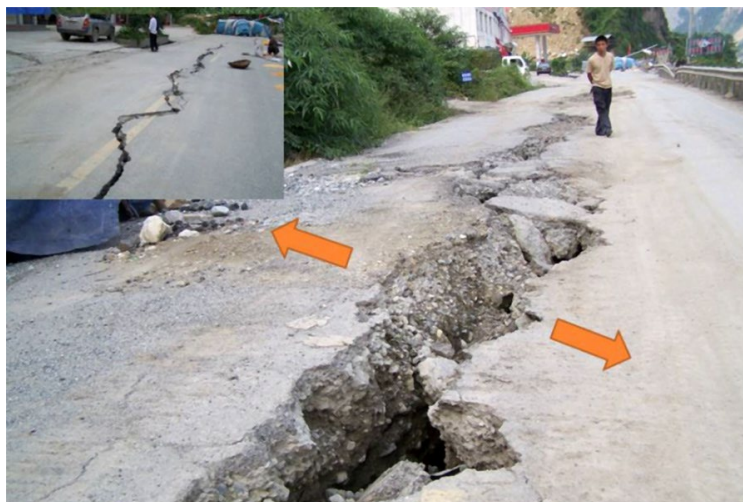
Figure 1.4 Tensile crack on the road surface due to the 2008 Wenchuan earthquake [6]
