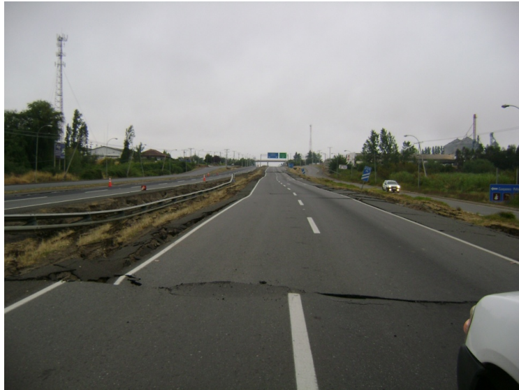
Figure 1.3 Shear failure, Chile (Lewis [7])
