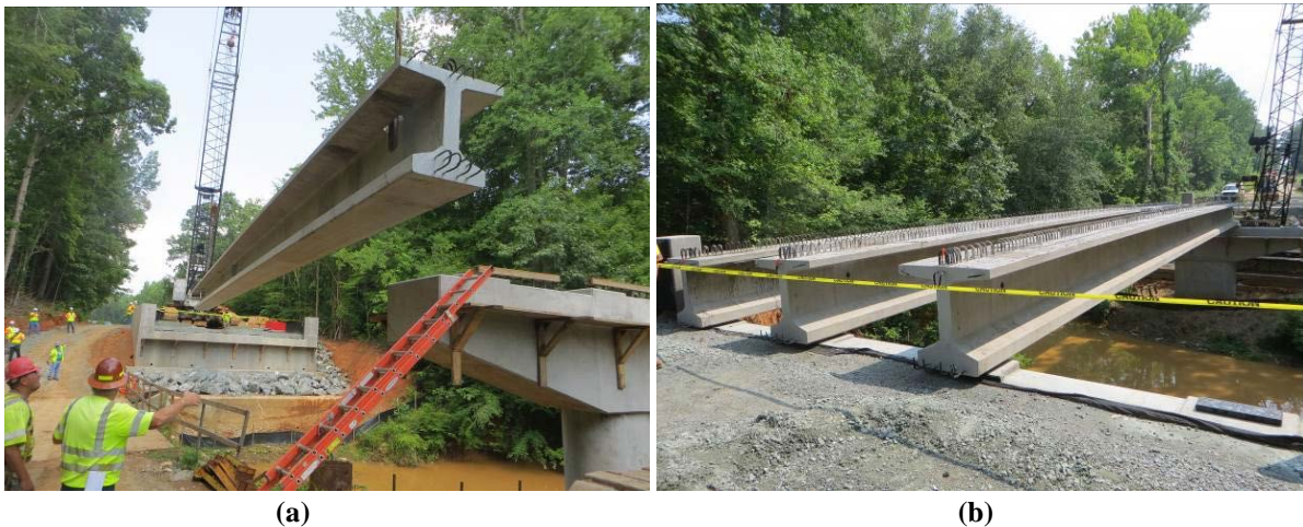
Figure 4. Bridge Construction: (a) beams being delivered to the jobsite and erection of first beam; (b) three beams in place
