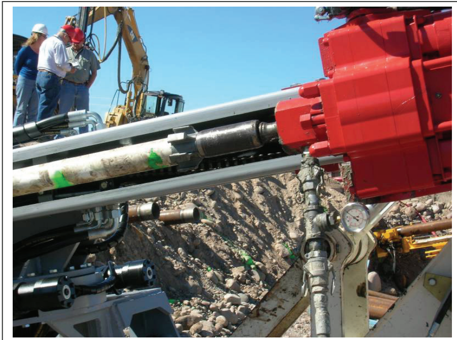
Figure 11. Photograph. Top hammer setup used for installation Methods B and C. Note the grout pressure gauge at the swivel and centralizer used to hold PVC in place.
