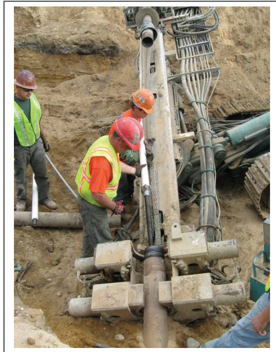
Figure 1. Photograph. Installation (Method A) of a solid bar at the Posillico Site.
