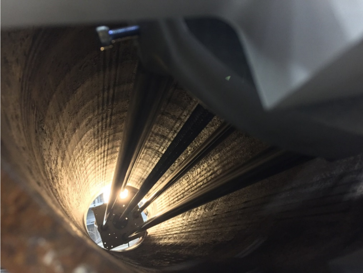
Figure 43. A photo of the inner surface of the 12-in steel pipes depicting an uneven inner surface.
