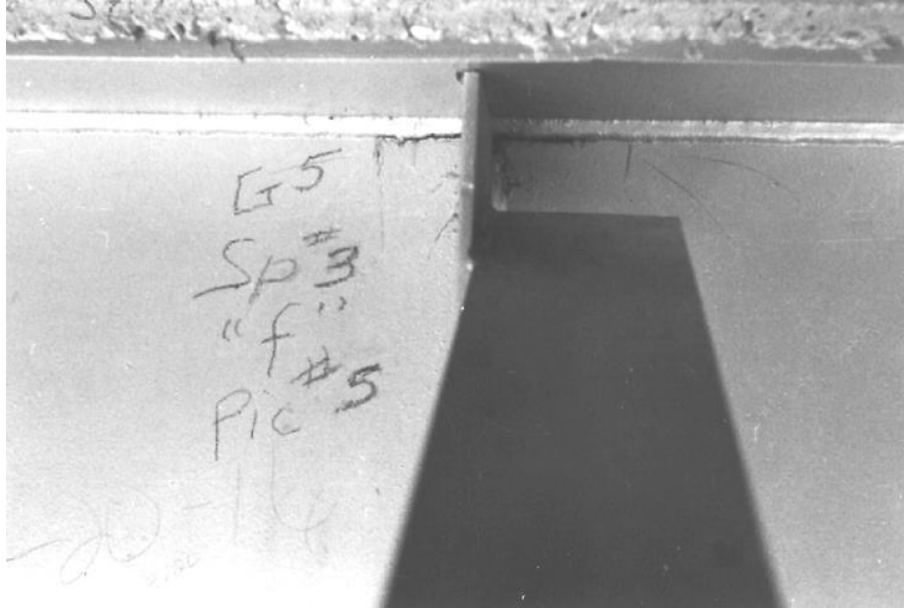
Figure 15 Fatigue Cracks in Web Gap of Diaphragm Connection Plate
