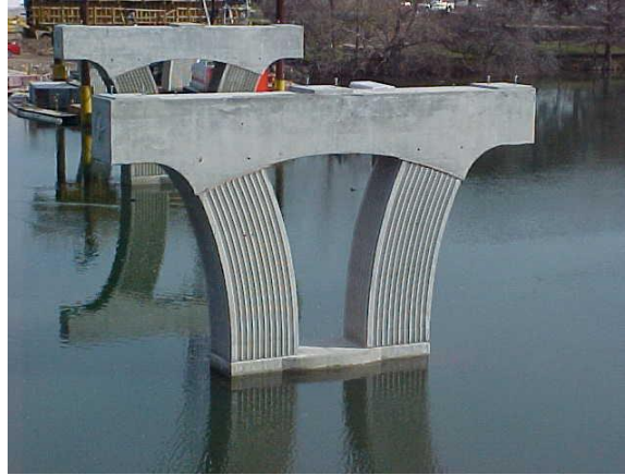
Figure 19 There can be a wide range of variations on the basic multi-column pier configuration, such as these piers with haunched pier caps and curved columns featuring formliner treatments for a pedestrian bridge.
