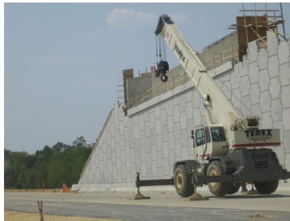
Figure 12 Conventional stub abutment with MSE retaining wall and wingwalls parallel to the abutment cap.
