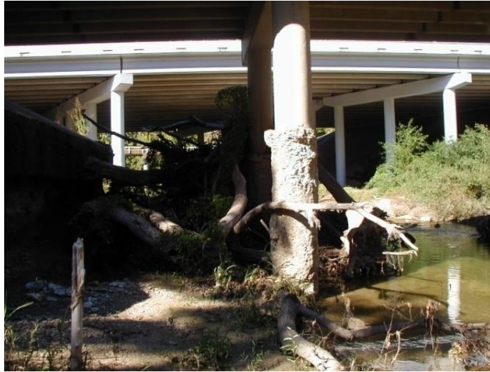
Figure 6 The effects of scour can be severe. Here a drilled shaft in a multicolumn bent has experienced over 6 feet of permanent (erosion) scour; during a flood event with higher velocity flow, there will be even more temporary (local pier) scour at this pier.
