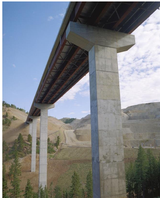
Figure 20 Single column hammerhead pier with very tall columns over a deep valley.
