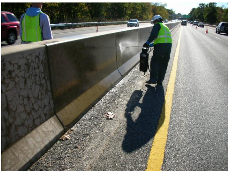
Figure 6. Photograph showing topical application of 40 percent-Silane Solution (solvent-based) to ASR-affected highway barrier in Massachusetts.
