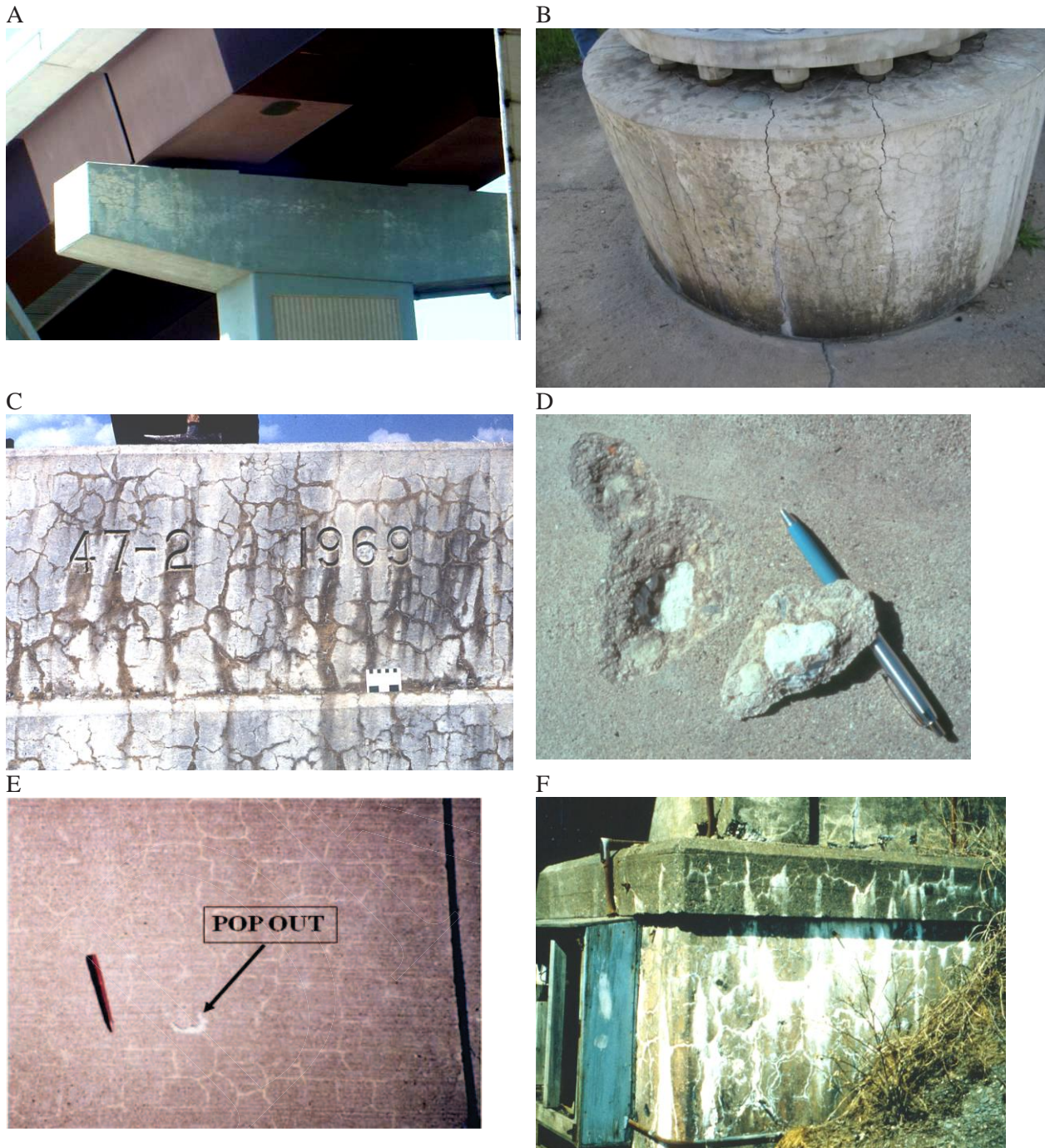
Figure A2. (A). Bent cap in relatively new bridge structure showing signs of ASR, primarily where direct access to moisture/rain prevails. (B). ASR cracking in drilled shaft supporting high-mast illumination pole. (C). Gel staining around cracks in the parapet wall of a bridge structure affected by ASR. (D). Pop-out created by the expansion of a frost-susceptible porous coarse aggregate particle. (E). ASR-induced pop-out in a concrete pavement incorporating highly-reactive aggregates; also noted pattern cracking (F). Efflorescence and exudations of alkali-silica gel at the surface of the concrete foundation of 25-year-old highway bridge affected by ASR.
