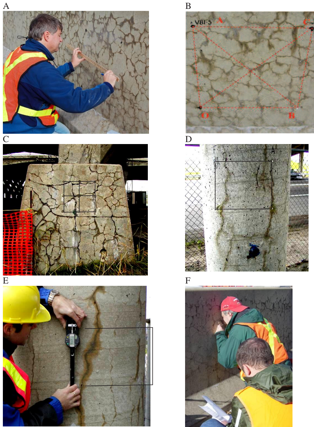
Figure B2. (A and B). Laying out of the reference grid on a concrete median barrier affected by ASR. (C). Four small reference grids are drawn on the exposed surface of the foundation block of reinforced concrete columns of a highway bridge structure affected by ASR. (D). Reference grid on the exposed surface of a reinforced concrete column of a highway bridge structure affected by ASR. (E). Expansion measurement at the surface of the above concrete column. (F). Cracking Index measurements.
