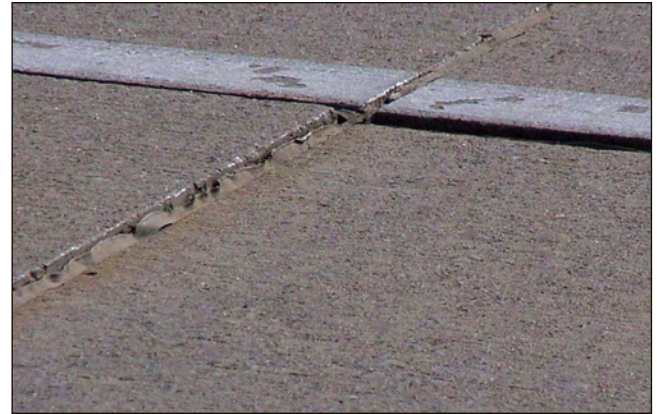
Figure 2-8. Faulting in jointed concrete pavement (ACPA)
