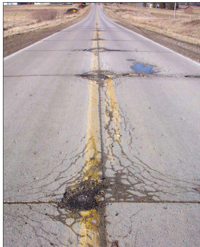
Figure 3-11. D-cracking (Grove, CP Tech Center)
