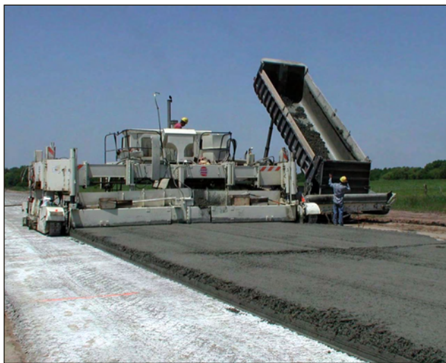
Figure 8-6. A belt placer/spreader ensures a consistent amount of concrete in front of the paver. (ACPA)
