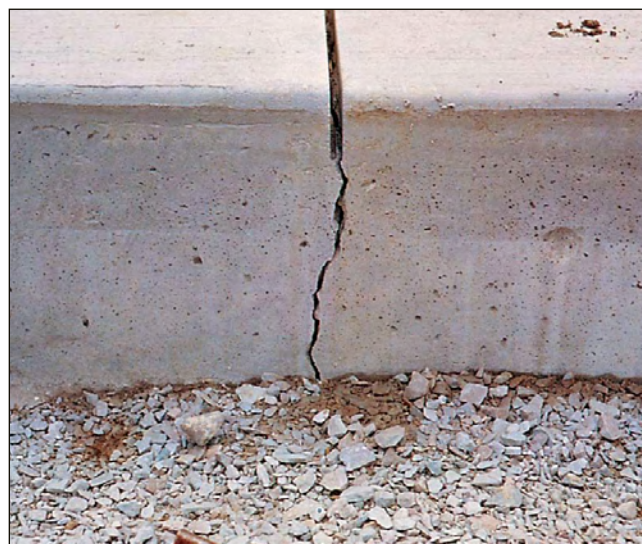
Figure 5-26. A saw cut that has cracked through as planned (PCA)
