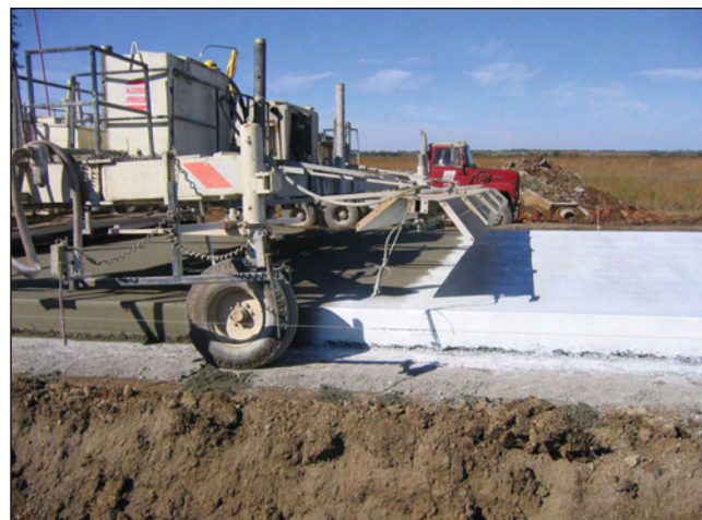
Figure 8-15. A curing machine coats both the top surface and sides of a slipform paving slab. (ACPA)
