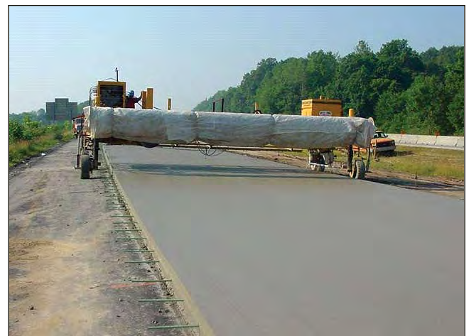
Figure 8-17. Plastic sheeting ready for placement to protect the fresh surface from rain (ACPA)
