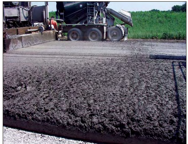
Figure 5-1. Segregated concrete (Hanson, Iowa DOT)
