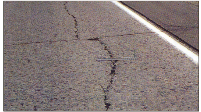
Figure 5-34. Random longitudinal crack
