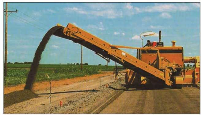
Figure 7-3. Autograder that references the string line and trims the subgrade material (ACPA)
