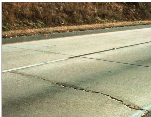
Figure 2-5. Transverse crack that represents structural distress (ACPA)
