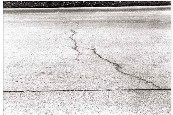
Figure 5-33. Random transverse crack
