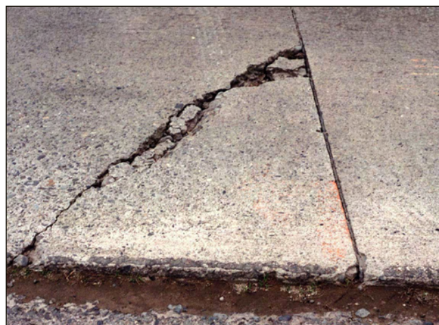
Figure 2-4. Corner cracking in jointed concrete pavement (ACPA)
