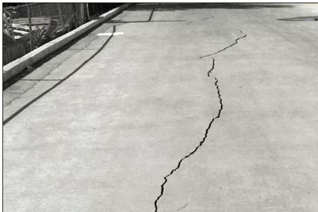
Figure 2-6. Longitudinal crack representing structural distress (ACPA)
