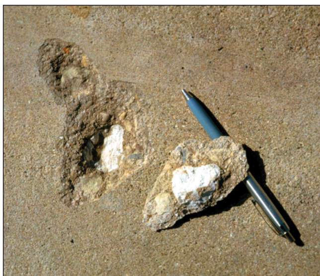
Figure 3-12. A popout at the surface of concrete (PCA)
