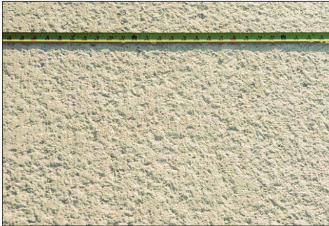
Figure 8-18. Typical scaling of concrete pavement due to rain on nondurable paste surface (ACPA 2003a)
