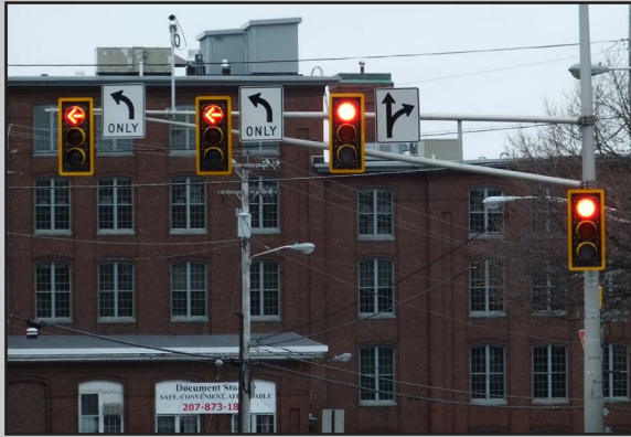
Exhibit 3: Signals with retroreflective backplates in the City of Nashua, New Hampshire. (Source: VHB)
