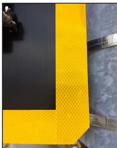
Exhibit 8: Installation details for retroreflective borders on backplates. The photo to the left shows where the backplate was cut along the bottom to fit around the signal head. The backplate was fastened to the signal housing to the left and right of the cut. The photo to the right shows a detail of the applied tape. (Source: VHB)
