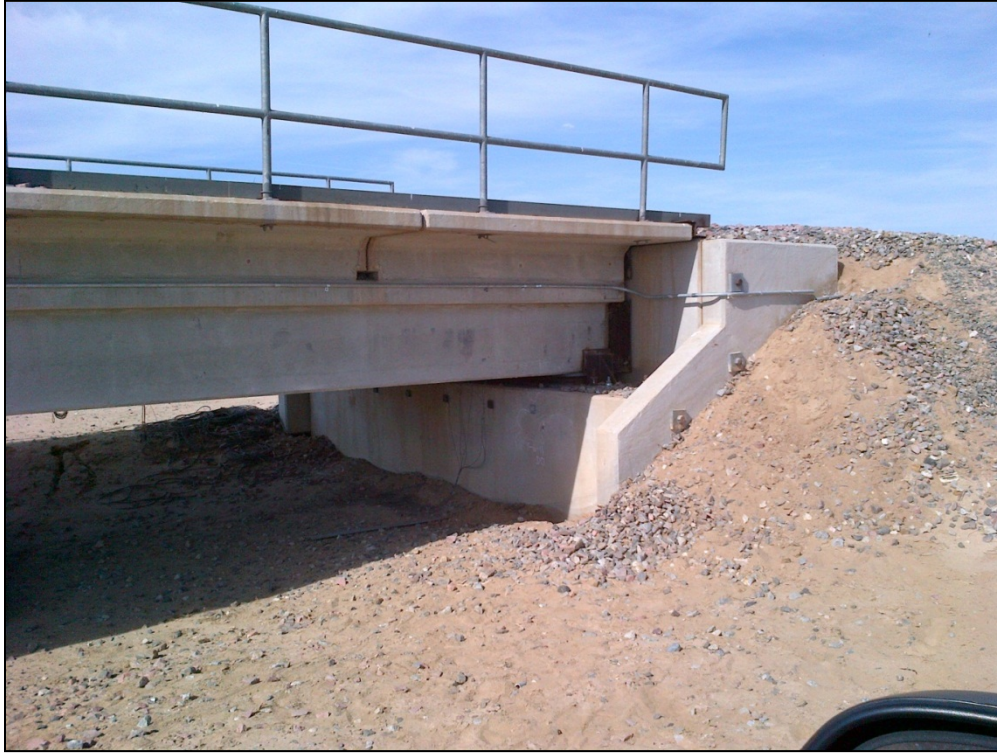
Figure 5: HTL Bridge with Fiber-Optic Conduit
