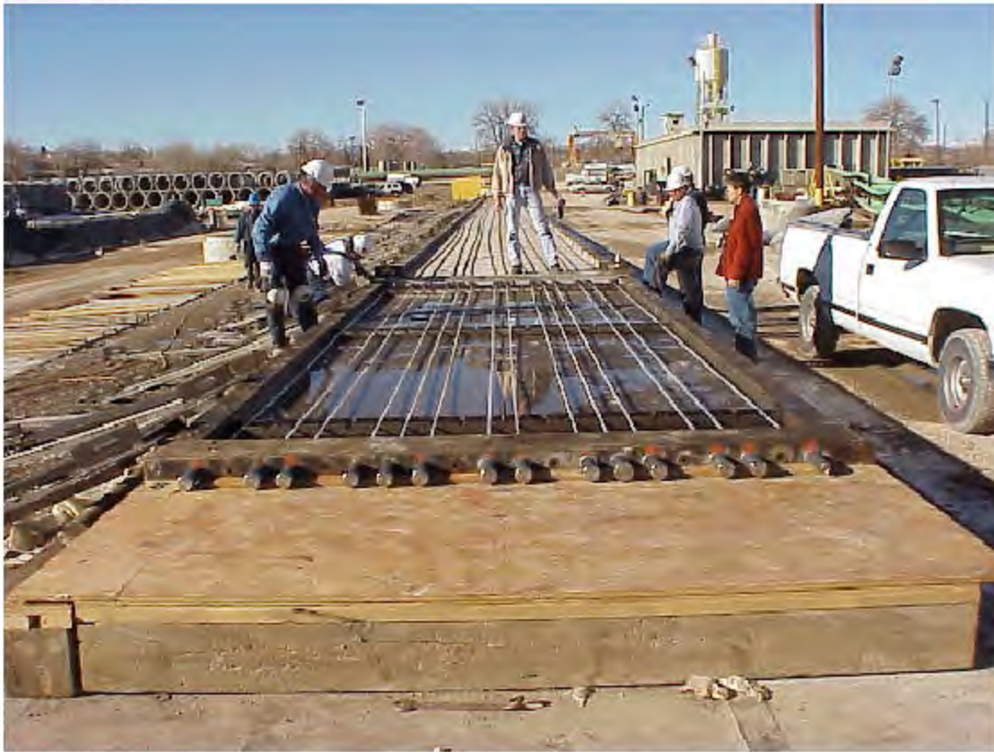
This photo shows a prestressed carbon fiber precast bridge panel. This project is the first time that CDOT has not used steel for reinforcement.
