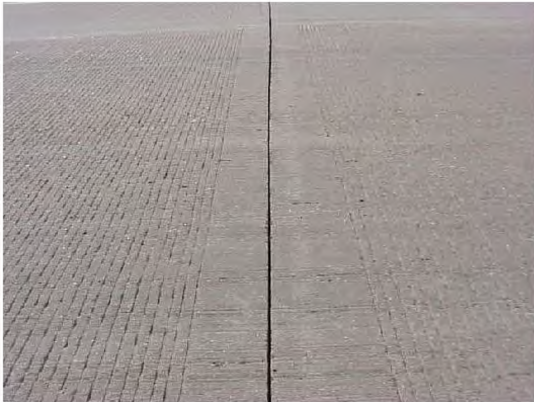
This concrete pavement joint has been left unsealed.
