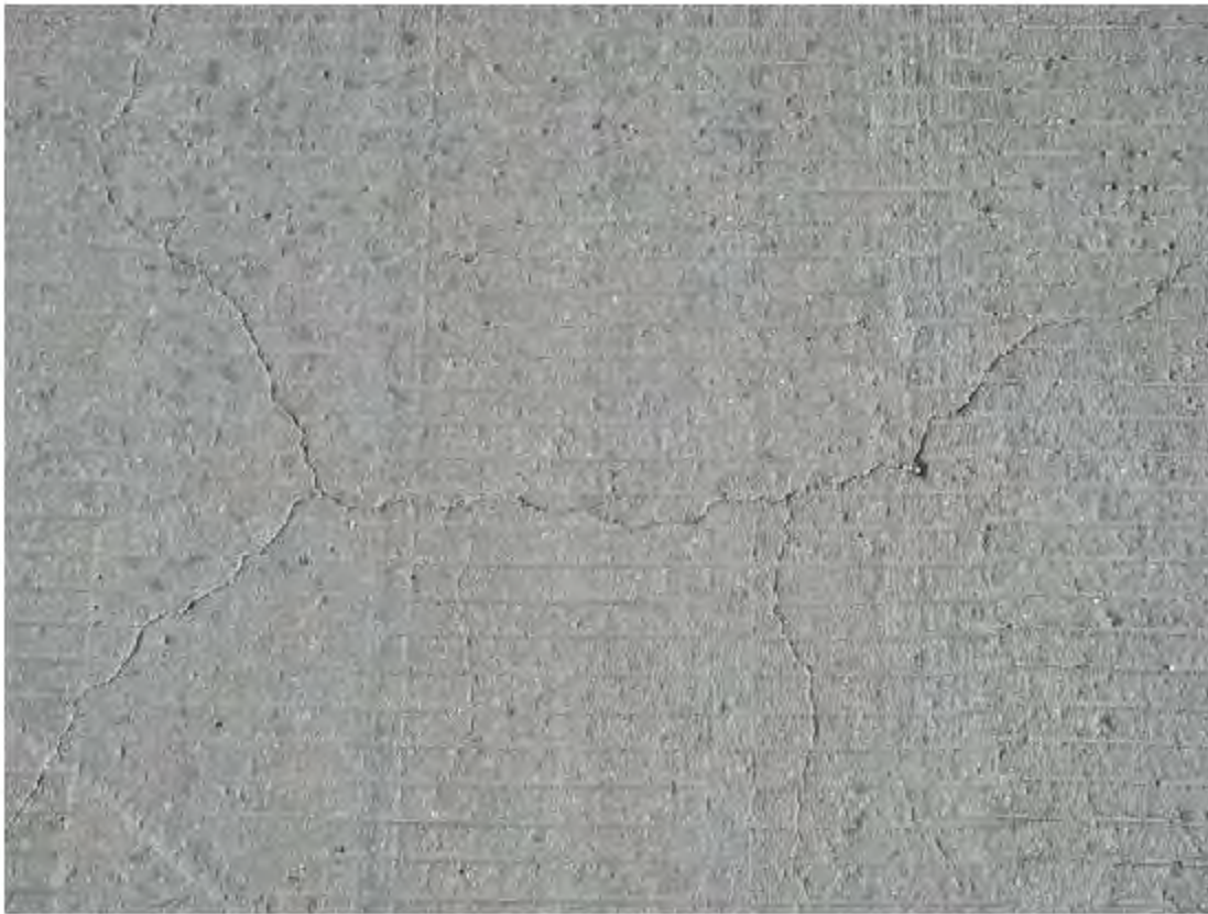
This bridge deck is showing extensive cracking.
