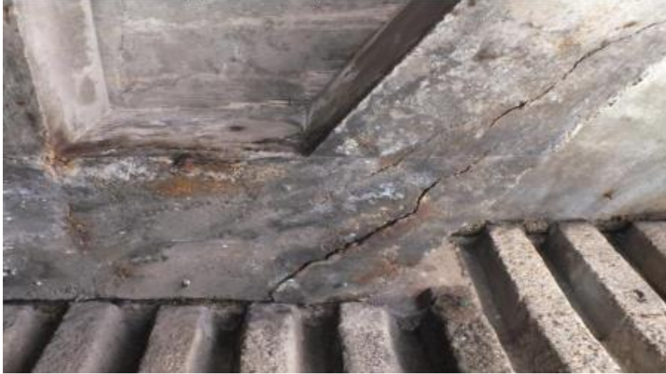
Figure 29: Widen cracks observed by Visual Testing (VT) method [82]
