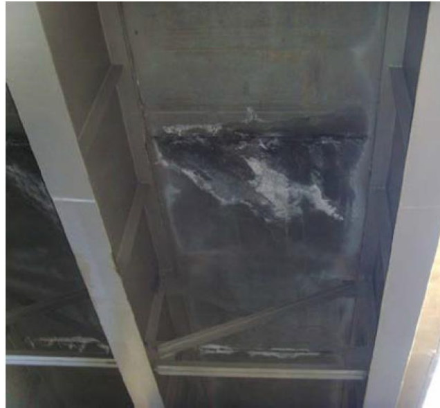
Figure 5: Typical joint leakage at deck panels (I-84 WB over Weber Canyon with welded-tie connections from 2009 inspection) [25]
