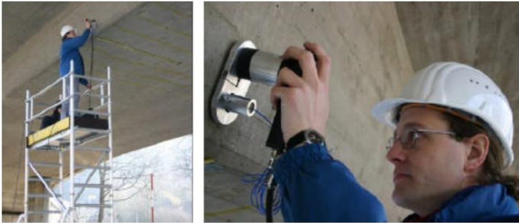
Figure 11: Void detection at bridge concrete by using IE method [44]
