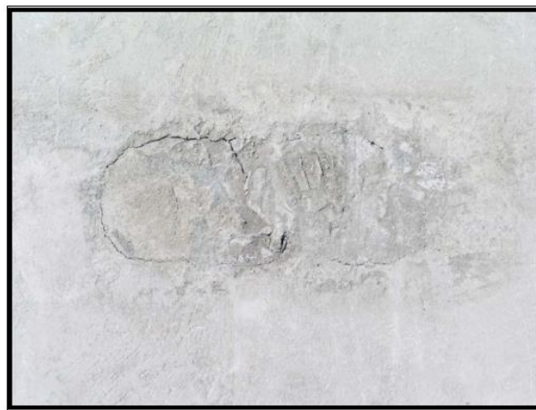
Figure 7: Shrinkage crack in the blackout type of ABC closure joint [22]
