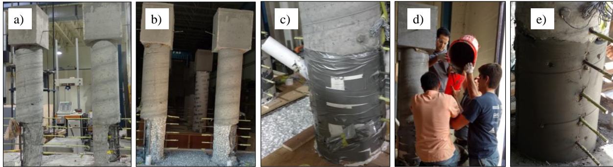
Figure 4. Repair Procedure: a) damaged part before repair, b) damaged part after sandblasting treatment, c) formwork for the repair plastering, d) casting UHPC, and e) damaged part after repair.
