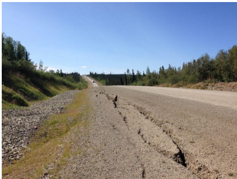
Figure 6: Example of Shoulder Rotation along an Alaskan Highway. 17
