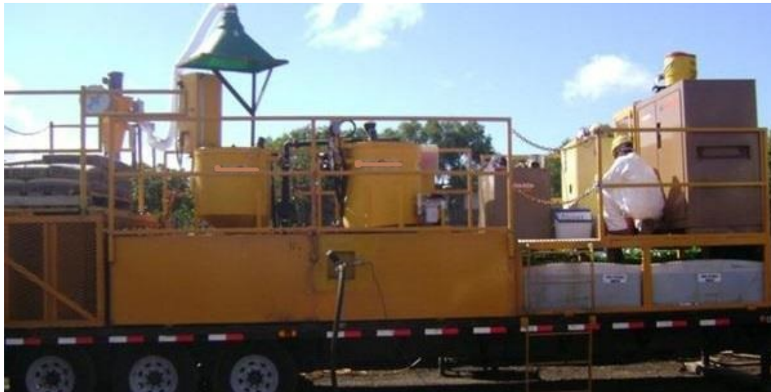
Figure 3.8: Grout plant with two tanks to maintain a continuous supply (courtesy of Applied Foundation Testing).
