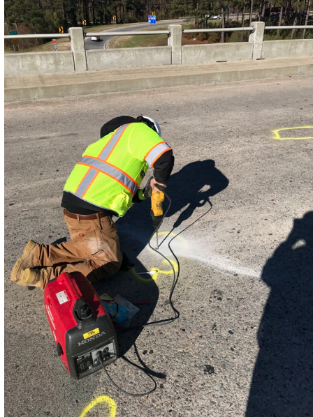
Figure 3.21: Drilling holes to collect concrete powder samples on US-21, Wilson Blvd. over I-20 bridge deck
