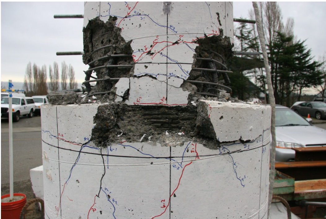
Figure 89. Photos. Specimen DS-1 column damage after cyclic testing.
