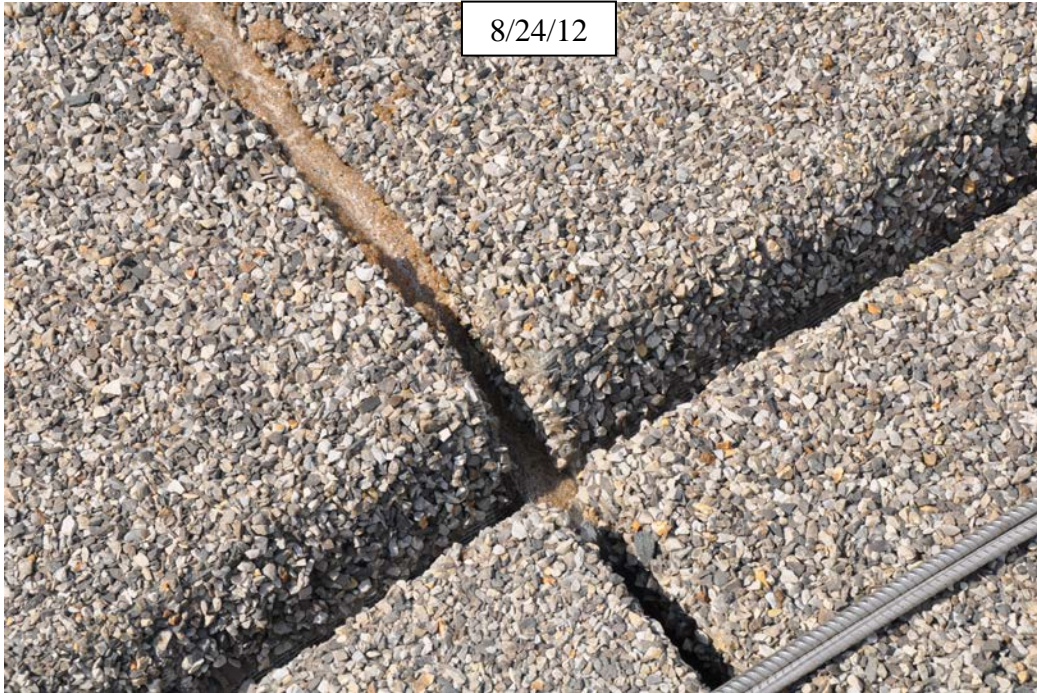
Figure 22. Photo. Install transverse rebar and epoxy grout in field joints. Thirty-six-inch #3 stainless rebar provides a positive tie across the centerline joint.
