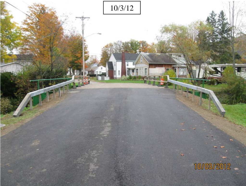
Figure 31. Photo. Install bridge railing posts, rails, and approach railing. Opened to traffic on 9/27/2012.
