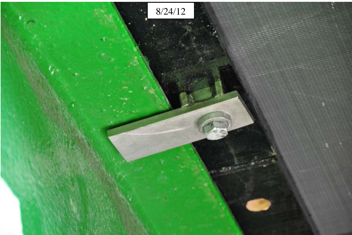
Figure 19. Photo. Installed clip. Methacrylate adhesive can be used to fill voids above or below prefabricated haunches to ensure uniform bearing. This was done on 9/4/2012.
