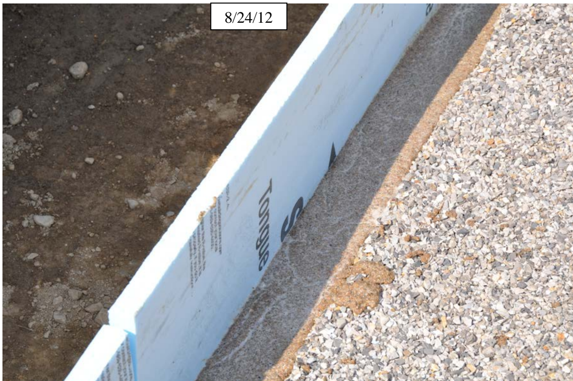
Figure 25. Photo. Install 1-inch foam backer board at bridge joint at each end of the deck to square up the end of the deck. Install epoxy grout in deck nosing at joints.
