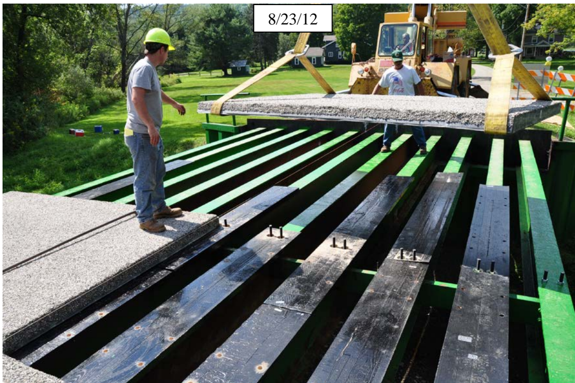
Figure 15. Photo. Place panels on top of prefabricated haunches. Note studs that make a fixed connection between the deck and stringers at midspan.
