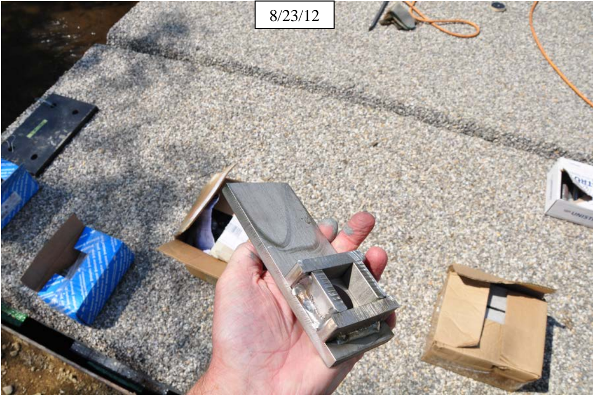
Figure 18. Photo. Secure panels with stainless steel clips and expansion bolts. Clip is shown.
