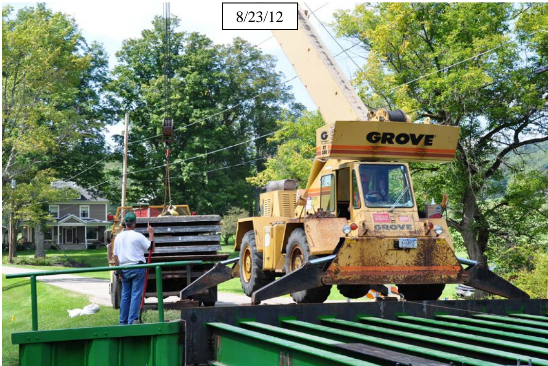
Figure 14. Photo. Situate crane and pick panels with two slings. Approximate panel weight is 20 psf, including wearing surface course 1. On this project, a panel weighed approximately 1,800 lb.
