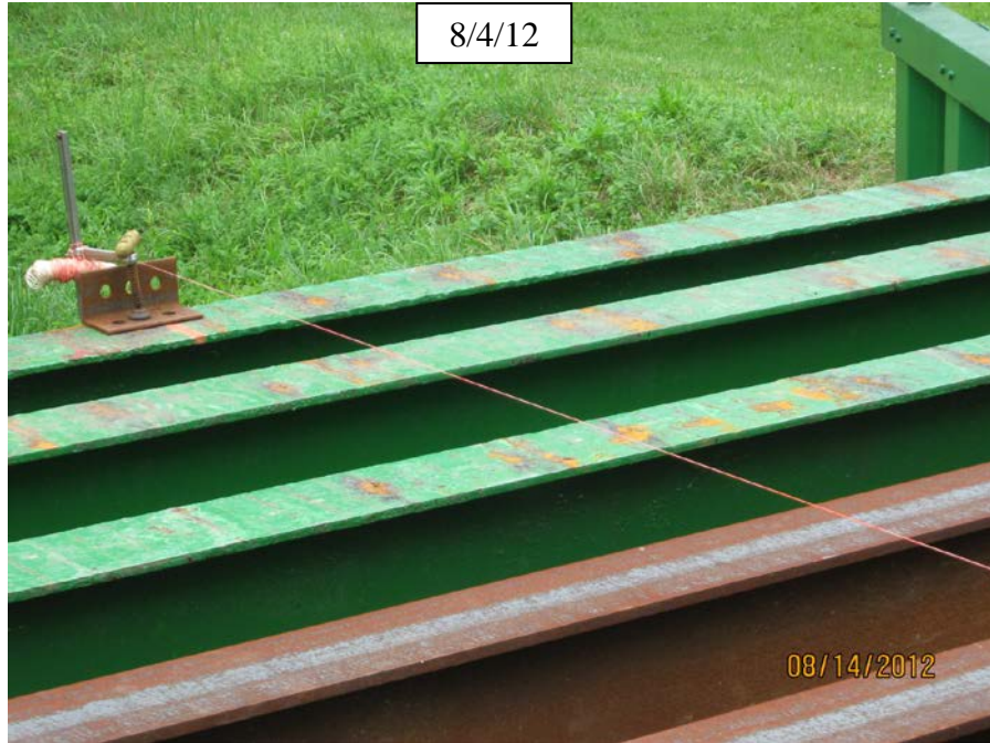
Figure 12. Photo. Stringline girders to determine if haunch corrections are needed. Note that the A588 stringer has replaced one that was corroded due to the previous open grating.
