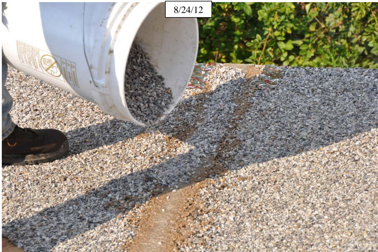
Figure 23. Photo. Embed clean, dry, angular aggregate on the surface of the epoxy-grout field joints.
