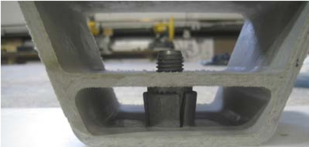
Figure 17. Photo. Secure panels with stainless steel clips and expansion bolts. Expansion bolt is shown.
