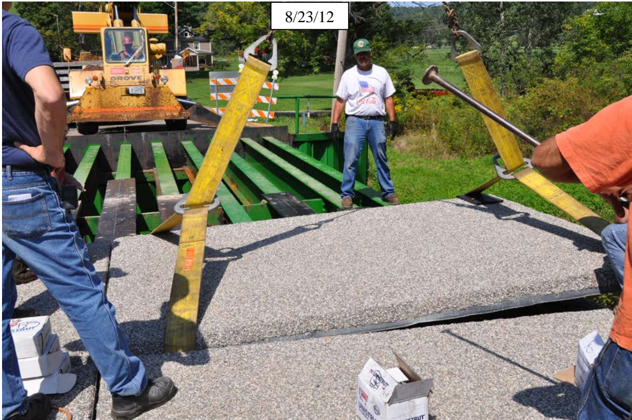
Figure 16. Photo. Place prefabricated deck panels so transverse field joints are as tight as possible, making fine adjustments with a steel road bar.
