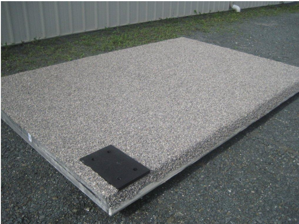
Figure 10. Photo. Adhesive and stone applied for course 1 of the wearing surface. Note the black prefabricated railing post pad and stone bonded to the sloped surface.
