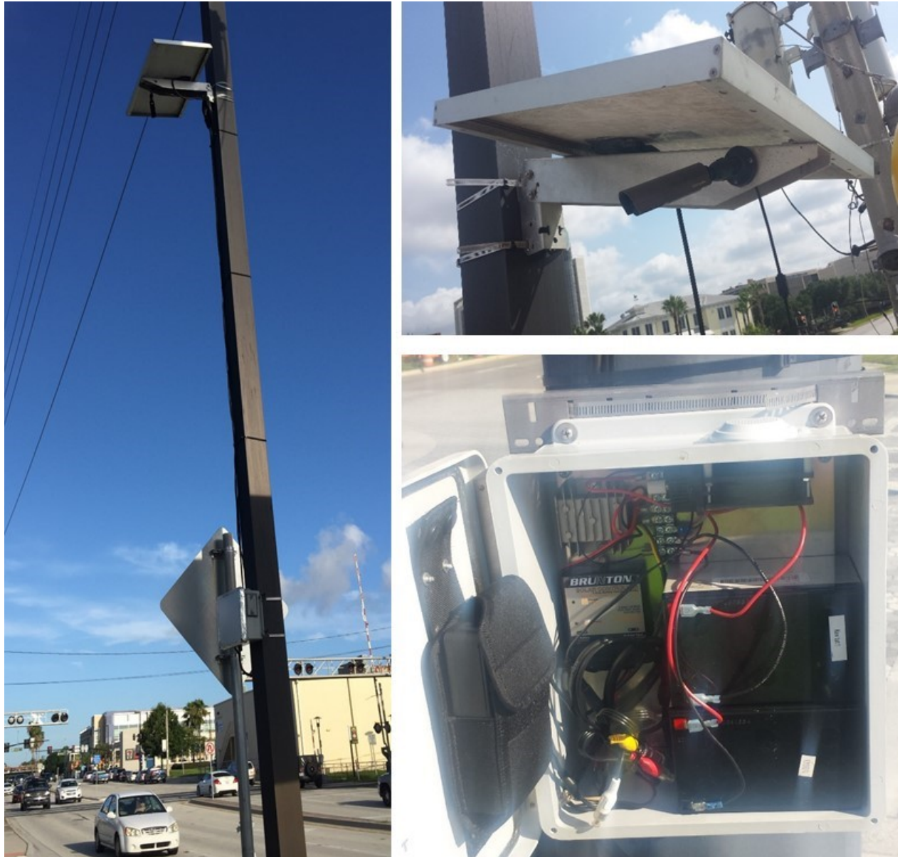
Figure 5. Video Data Collection System at East Princeton Street
