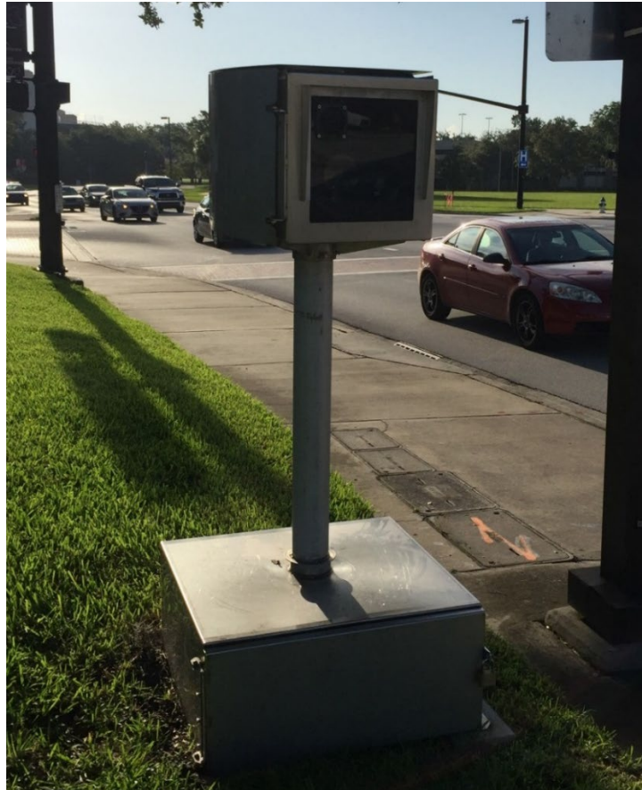
Figure 7. Photo Enforcement System at East Princeton Street
