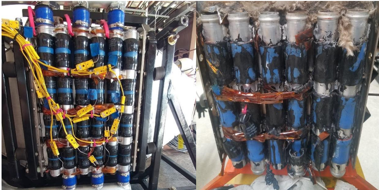
Figure 61, 62. Before and After Heat Shrink Hose Clamps Melted
