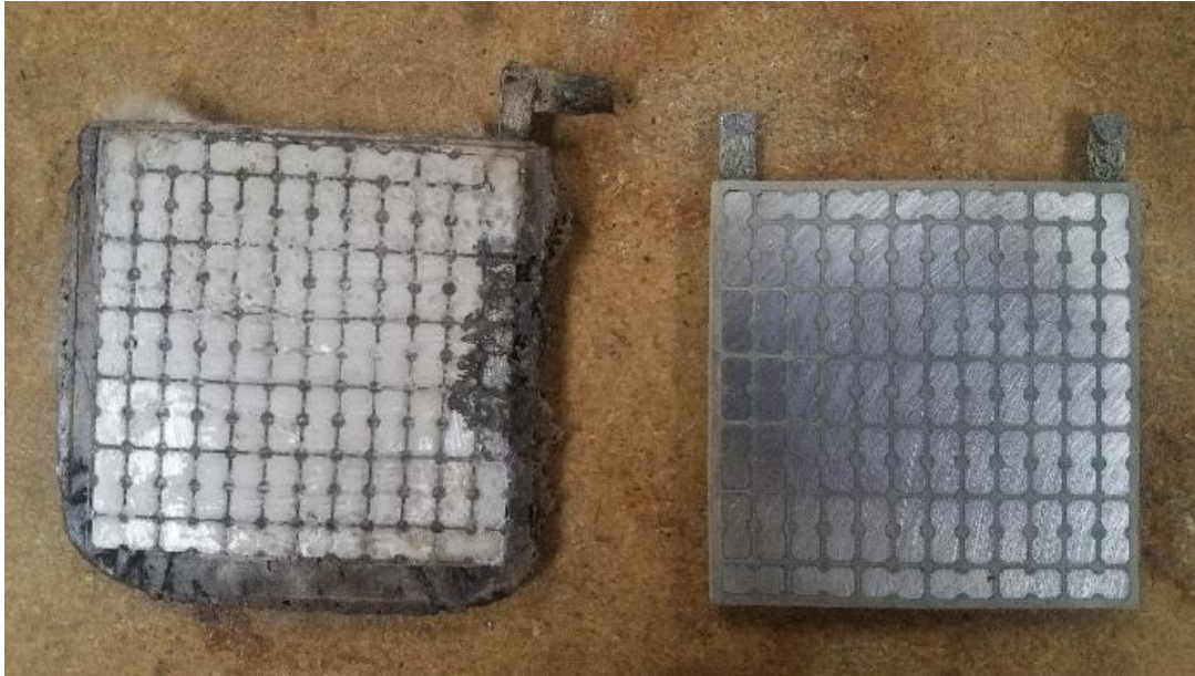
Figure 68. Overheated Module and New Module
