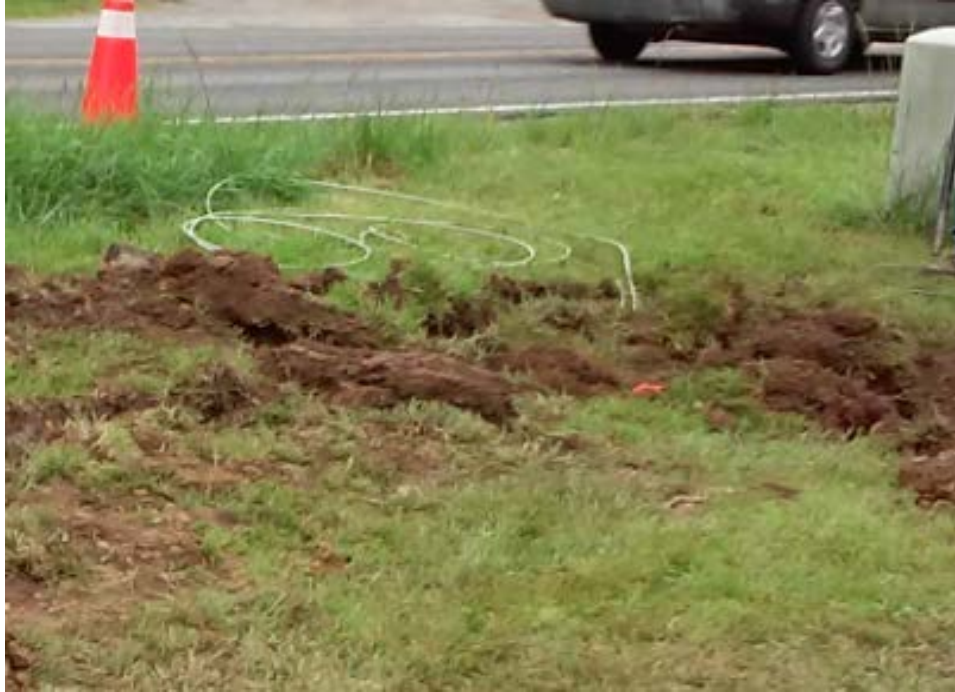
Figure 7. Lead-in Cables That Connect to the Processor Enclosure.
