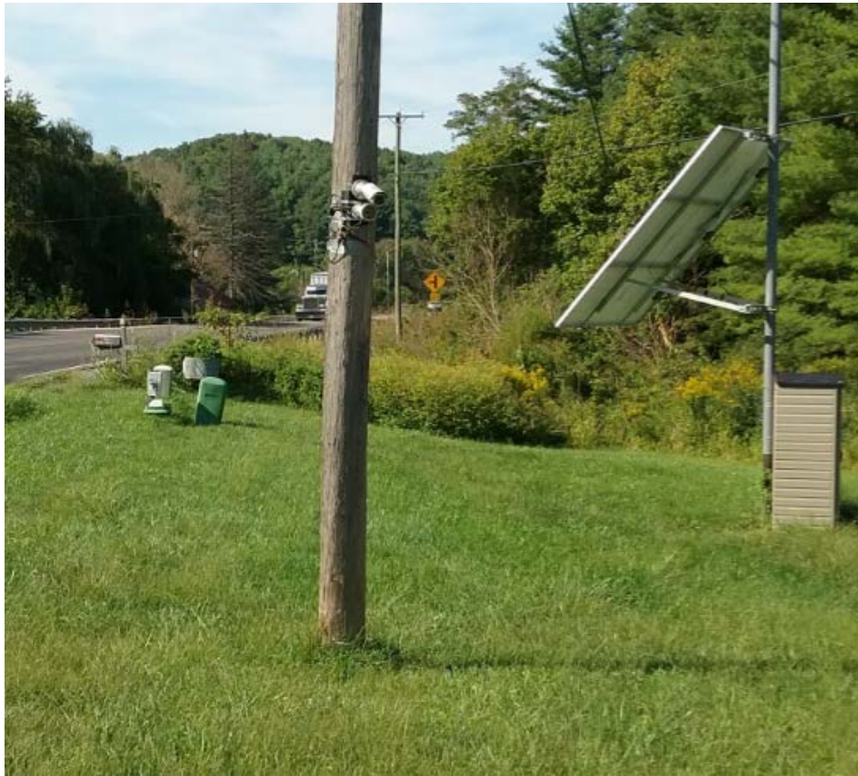
Figure 12. Surveillance Camera (Top) and Illuminator Used for Cable/Site Monitoring. The Solar Power System (Far Right) and Processor Enclosure (in the Background) are also Shown.
