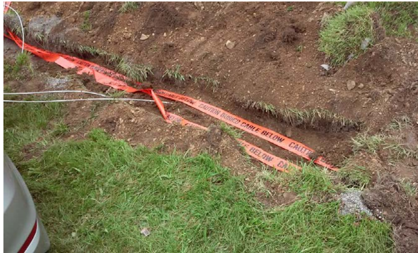
Figure 5. Trench Being Backfilled After Cables were Placed on the Crushed Stone Base.
