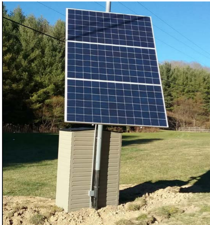
Figure 9. Solar Photo-voltaic System Supplying Power to the Buried Cable and Surveillance Equipment.
