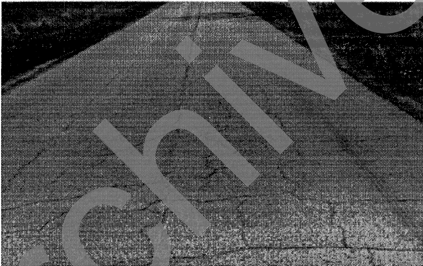
Figure 2-4. Example of intermediate-sized block cracking. (1)
