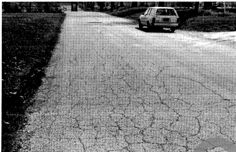
Figure 2-7. Example of typical alligator cracking pattern. (1)
