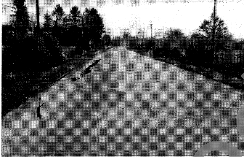
Figure 2-5. Example of slight to moderate rutting. (1)
