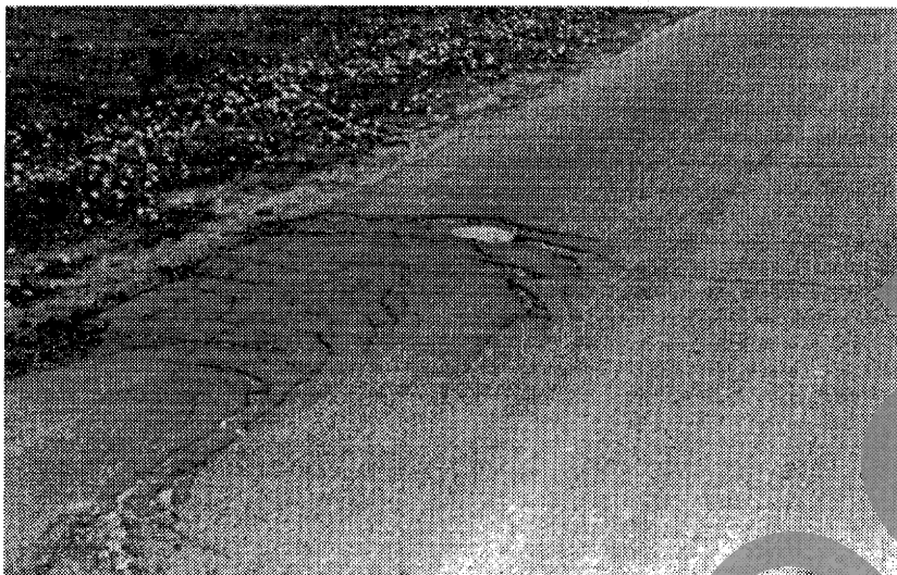
Figure 2-3. Example of slippage cracking. (1)
