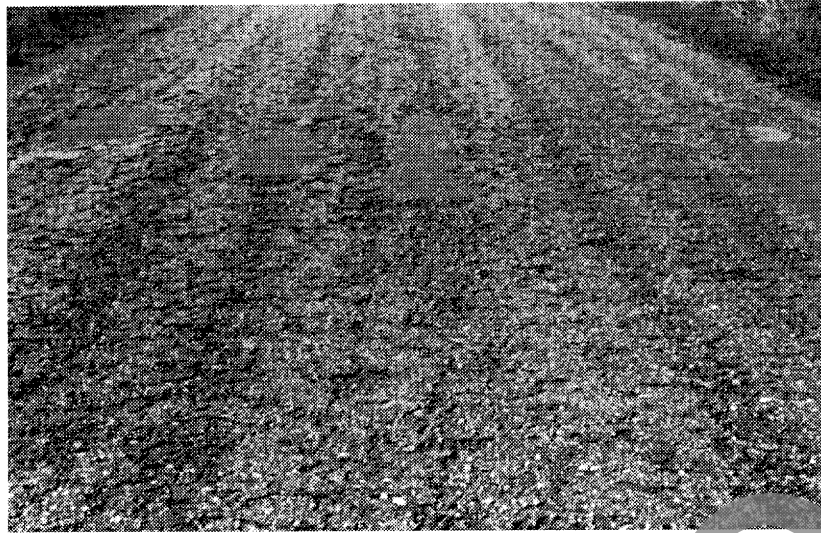
Figure 2-1. Example of severe surface ravelling. (1)
