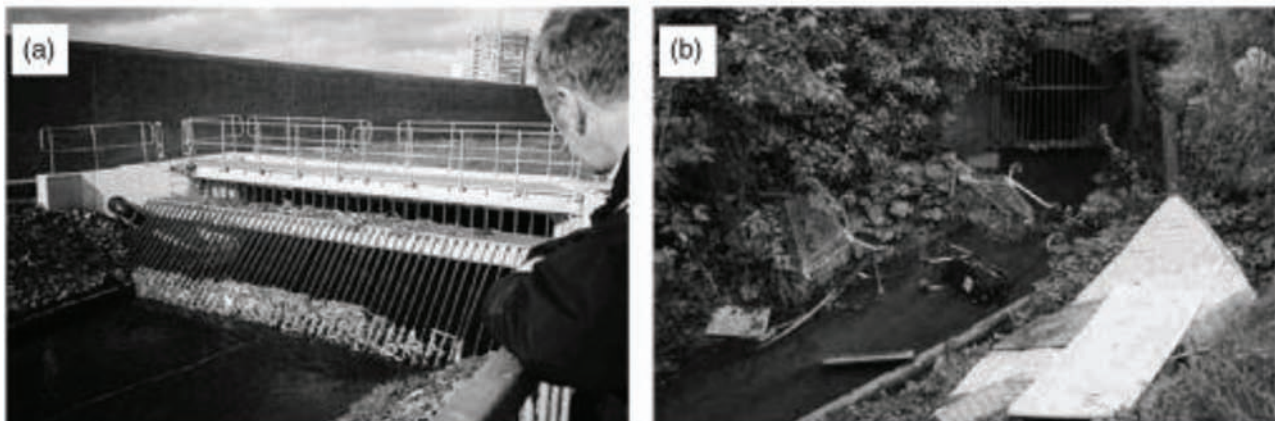
Figure 5.1 (a) Screen protecting inlet to large culvert with leaf-litter accumulation; (b) screen protecting culvert inlet on small channel with fly-tipped waste.
